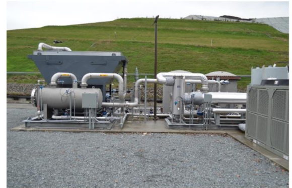
Picture 2 – Chiller & Dryer Skid
