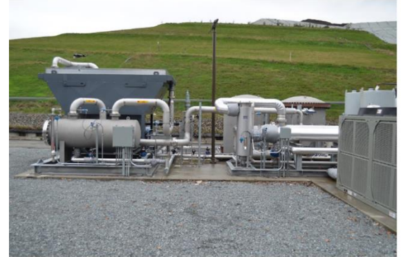
Picture 2 – Chiller & Dryer Skid
