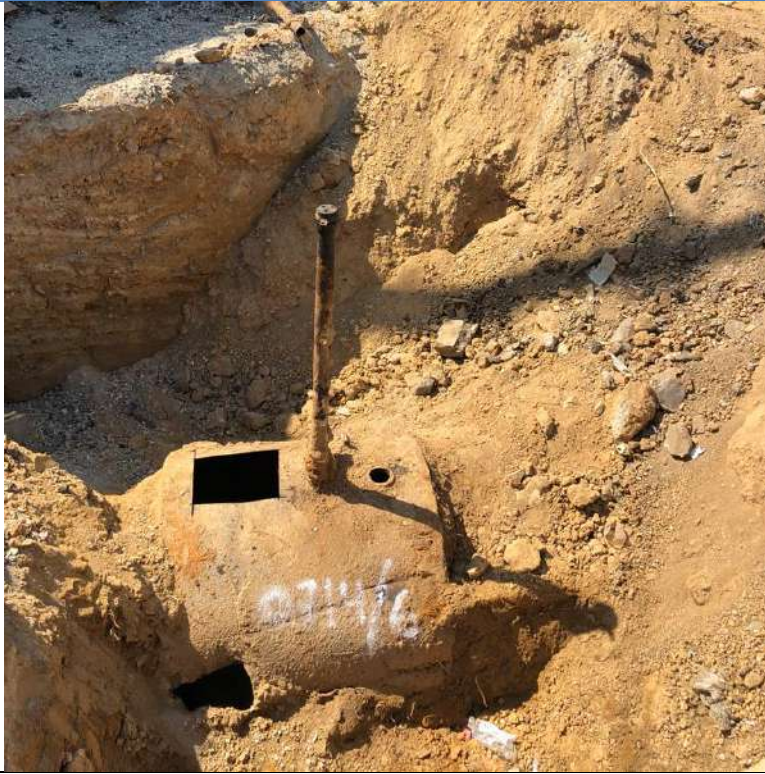
PHOTO 7: UST No. 6 certified clean and labeled (07/14/22).
