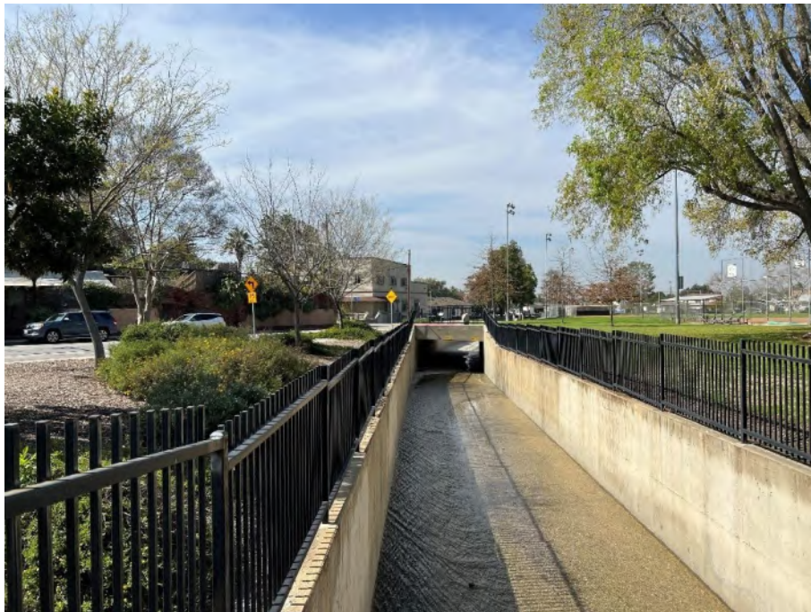
Exhibit 5. Overview of Little Dalton Wash pedestrian crossing from East Dalton Avenue to Skatepark, facing southwest.
