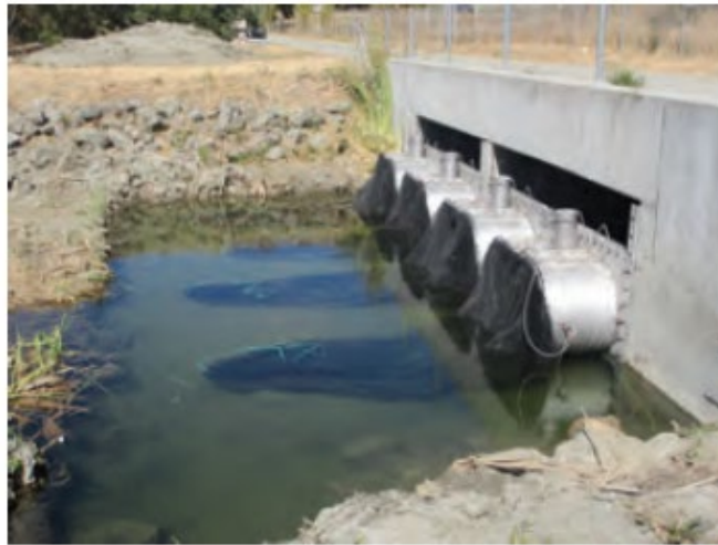
Representative Image 4. Example of End-of-Pipe Netting System
