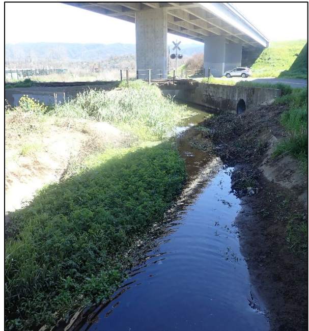
Photo 8. Looking downstream from box culvert at UK.21. In the background, a culvert that runs under Ford Road can be seen. Note the concrete lined slopes (April 4, 2023).
