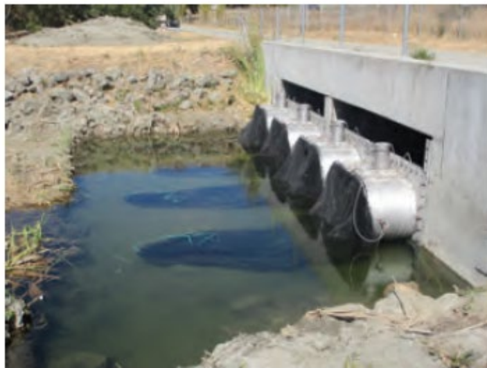
Figure 5. Example of End-of-Pipe Netting System
