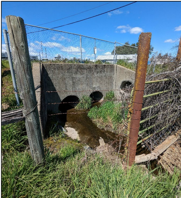
Photo 3. Wingwall at UK.10. A fence and gate are along the private property boundary (April 4, 2023).
