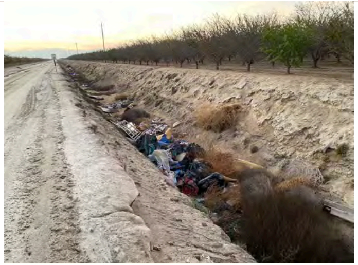
Large amount of debris in canal
