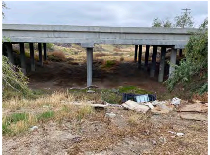
drainage under CA180; no culvert visible; debris dump off road fill
