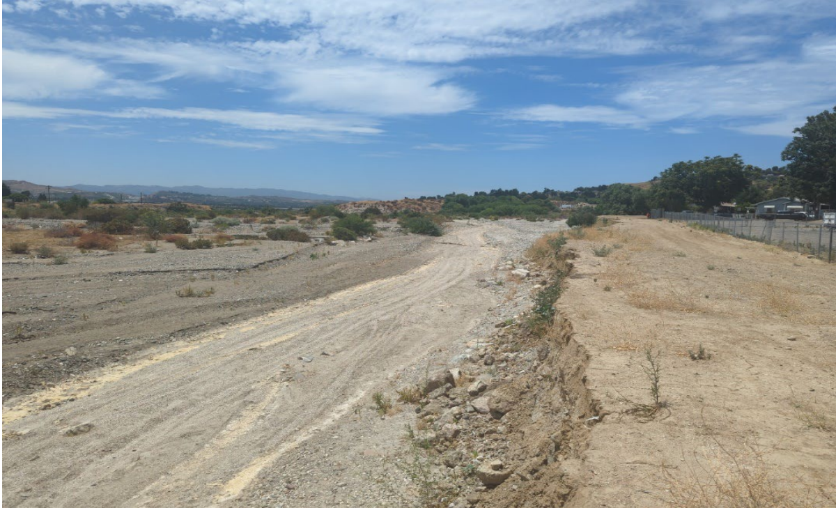
Photograph 15. Photo Point 15. View of the northern bank of the SCR in the central portion of the APE where soil cement bank protection is proposed, facing west. Note unstable, eroding bank and compacted, barren soils immediately north of the bank (August 1, 2023).
