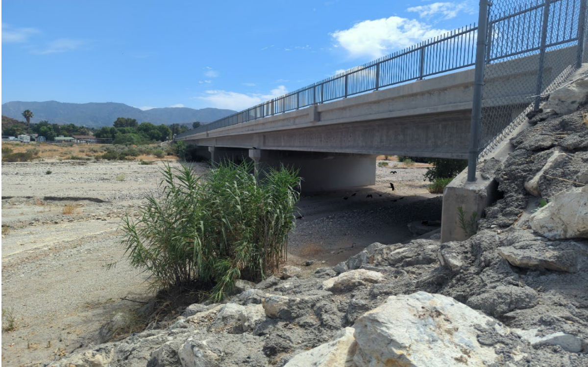
Photograph 25. Photo Point 25. View of the northern bank of the SCR to the east of the Sand Canyon Bridge, facing southwest. Note presence of rip-rap along the northern bank (August 1, 2023).
