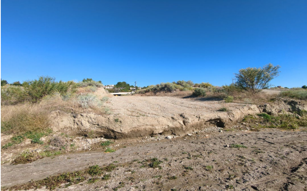
Photograph 35. Photo Point 35. View of an existing access road and the SCR channel in the southwestern portion of the APE near the proposed staging area, facing north (October 16, 2023).
