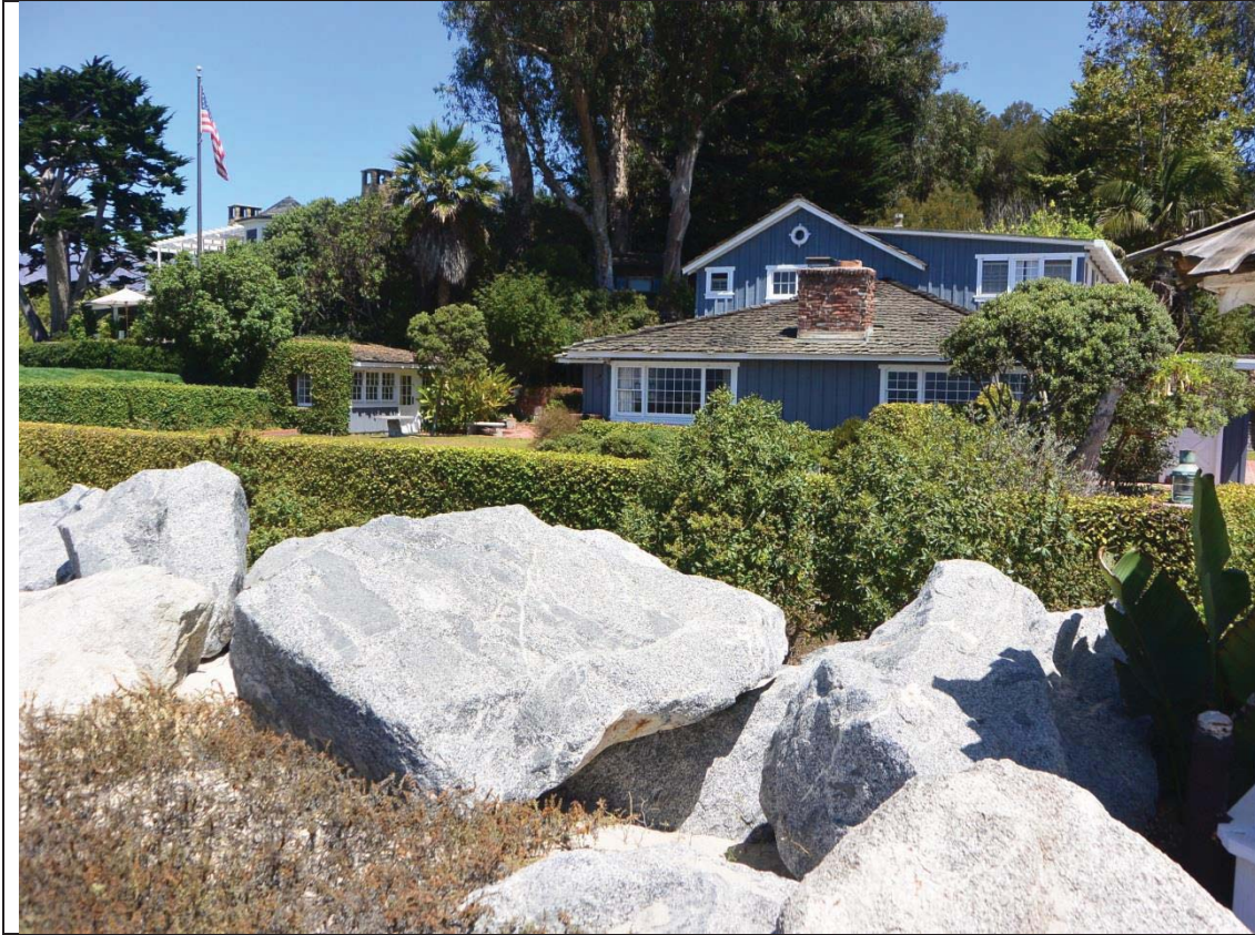
Photo 7. Sea wall in southern portion of property on the beach, protecting the two story single family residence (view looking north taken August 2, 2021)
