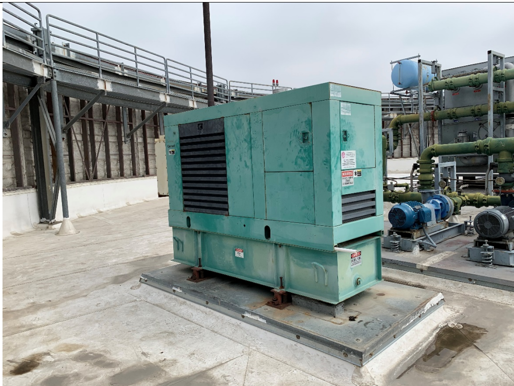
Photo #4 View of the backup diesel fuel generator located on the roof of the 5665 Plaza Drive building.
