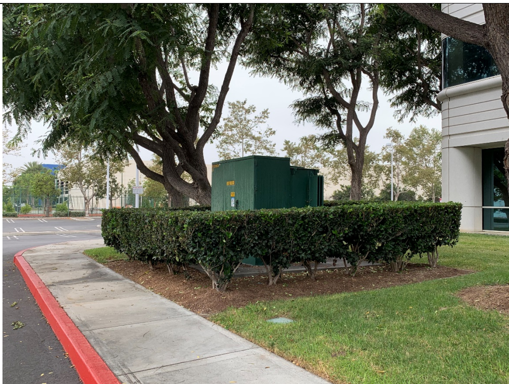
Photo #2 View of the pad-mounted transformer located in the southwestern corner of the building exterior.
