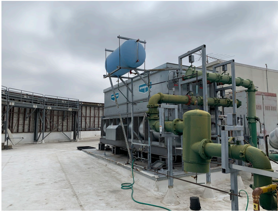
Photo #5 View of the roof mounted chiller on the 5665 Plaza Drive building.
