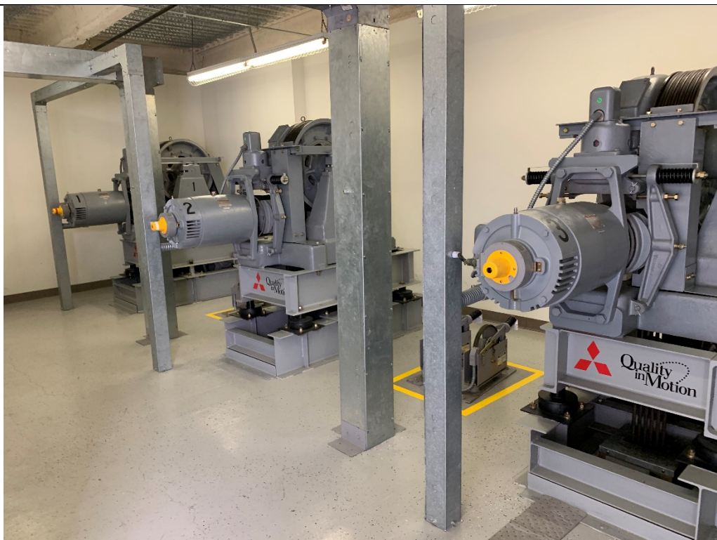
Photo #6 View of the elevator maintenance room on the roof of the 5665 Plaza Drive building.
