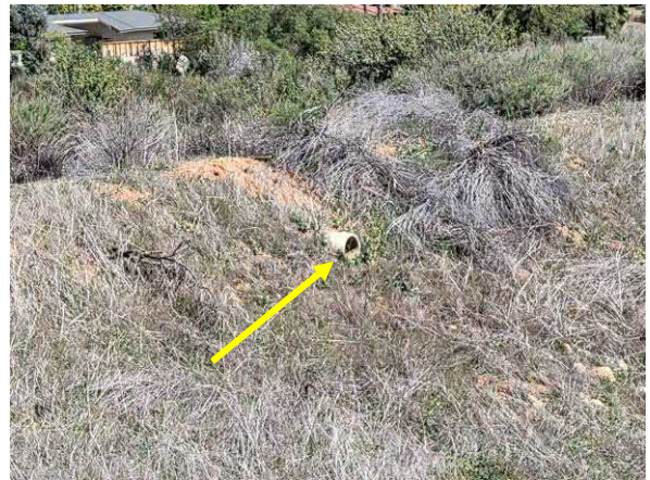
Photo #4 View of storm water drainage pipe (concrete), located on the central portion of the site.
