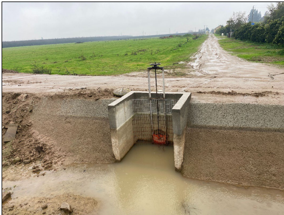
Figure 31. Turnout on Hansen Ditch segment with concrete headgate and modern manual hoist gate, facing slightly south.
