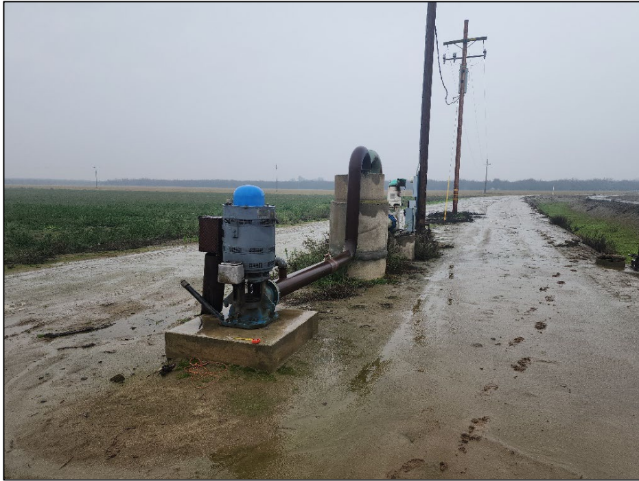
Figure 27. Pump and standpipe near turnout 23, facing southeast.
