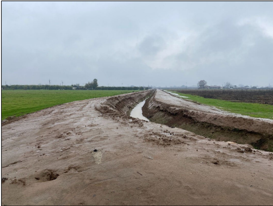
Figure 32. View of Hansen Ditch (segment) at curve near the end of the segment, facing west.
