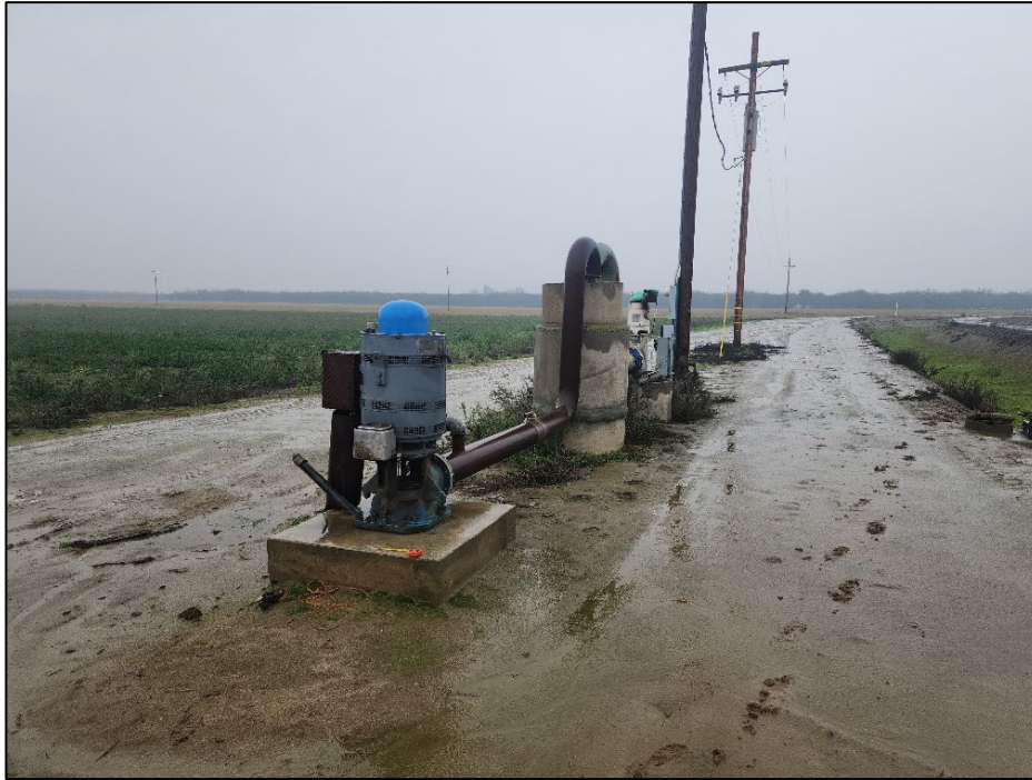
Figure 29. Pump and standpipe near turnout 23, facing southeast.
