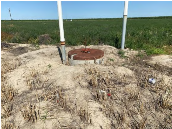
7. Irrigation standpipe valve on central portion of Subject Property near the south boundary
