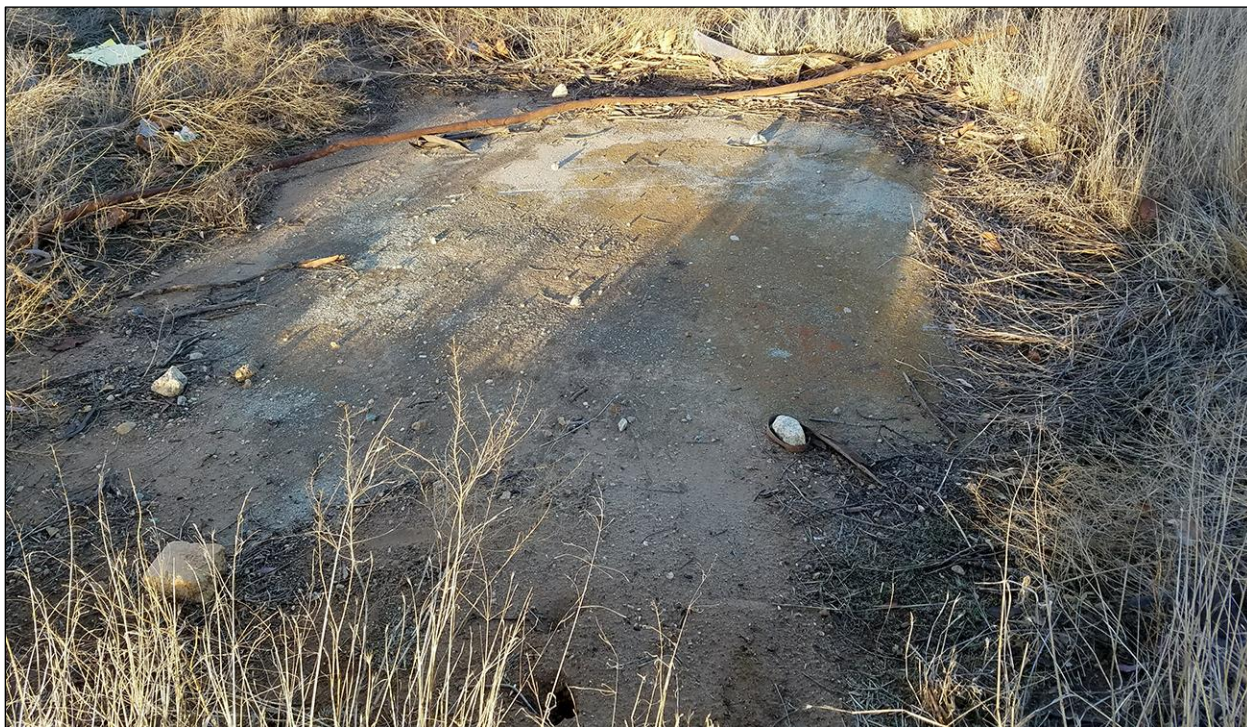
Figure 10. Remnants of concrete slab foundation in the project area. (Photograph taken on January 15, 2018)
