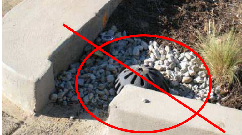
Figure 6: Incorrect Placement of an Overflow Inlet.
