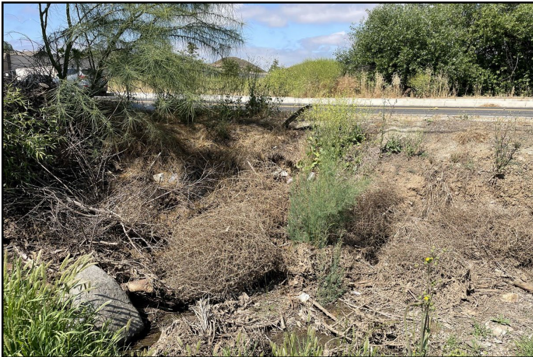
PHOTOGRAPH 4 View of Vegetation Debris at Culvert Inlet Upstream of Goetz Road
