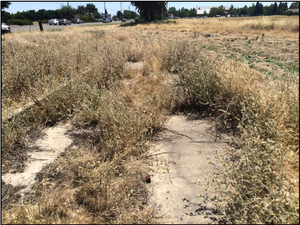
Figure 9. P-34-005386/CA-SAC-001278H, F-002 concrete structure pad densely overgrown with weeds, view south
