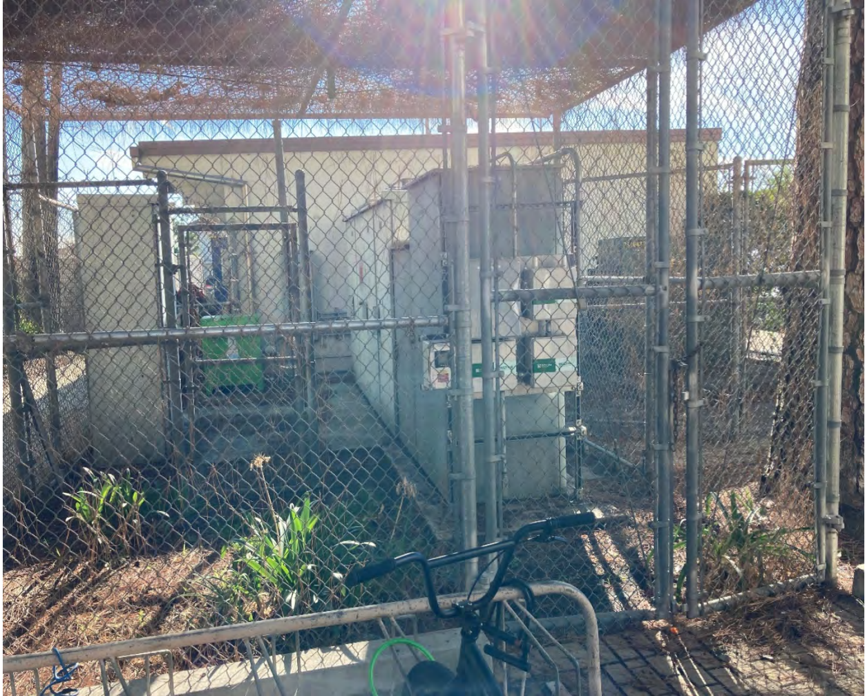
Campus transformers/ SCE utility boxes located south end of campus.
