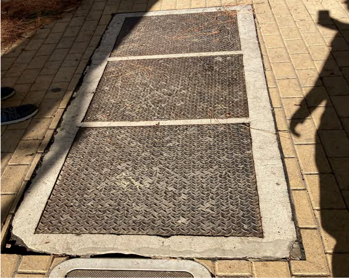
3-stage clarifier located adjacent to building 300.
