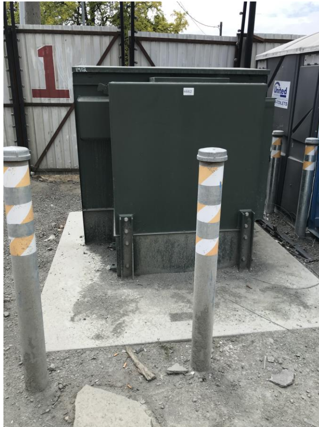
Photograph 4: Transformer on Pick-N-Pull portion of the Site.
