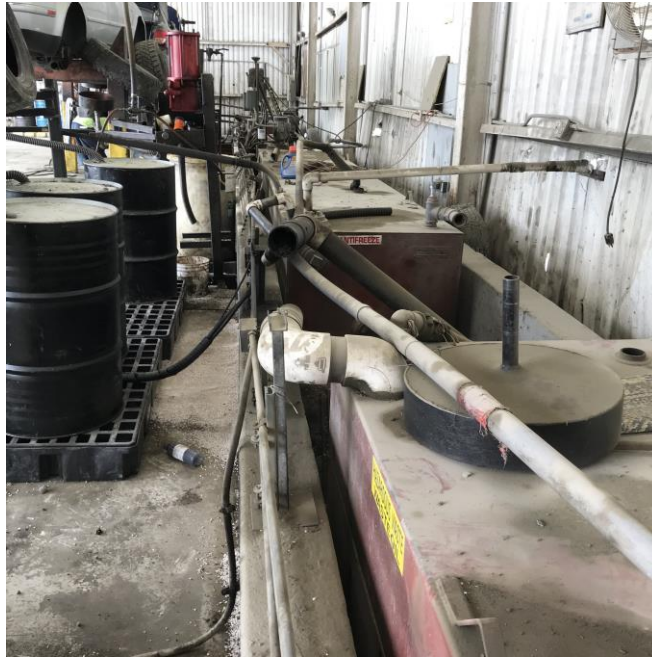
Photograph 13: Aboveground storage tanks in fluid-removal structure on Pick-N-Pull portion of the Site.
