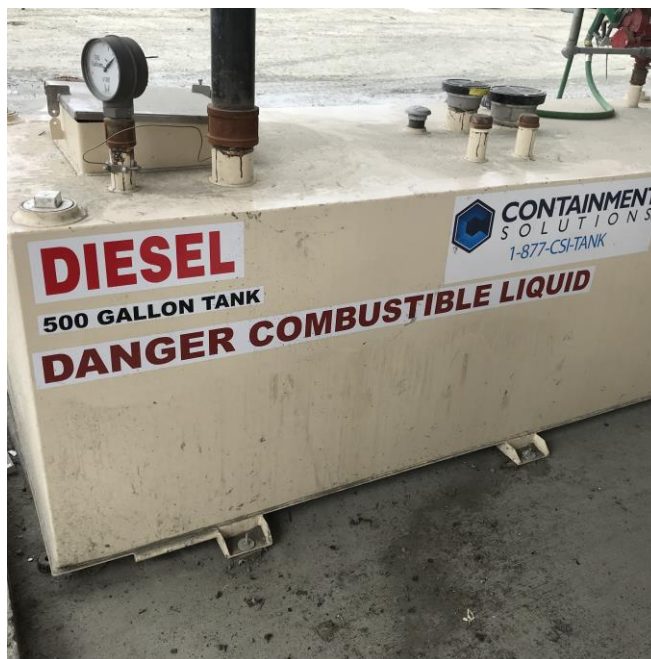
Photograph 12: Diesel aboveground storage tank in fluid-removal structure on Pick-N-Pull portion of the Site.
