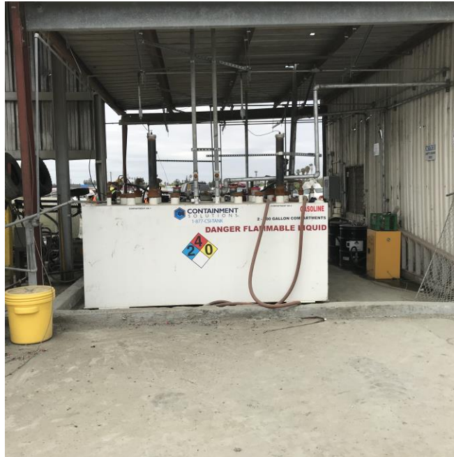
Photograph 11: Gasoline aboveground storage tank in fluid-removal structure on Pick-N-Pull portion of the Site.
