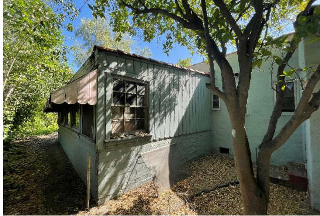
Figure 9F. Western Façade (rumpus room addition; view northeast) SOURCE: Sapphos Environmental, Inc., 2022
