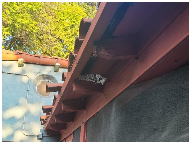
Figure 6I. Primary Façade (porch roof wood rot; view west) SOURCE: Sapphos Environmental, Inc., 2022
