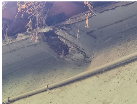
Western Façade (rafter, wood rot)
