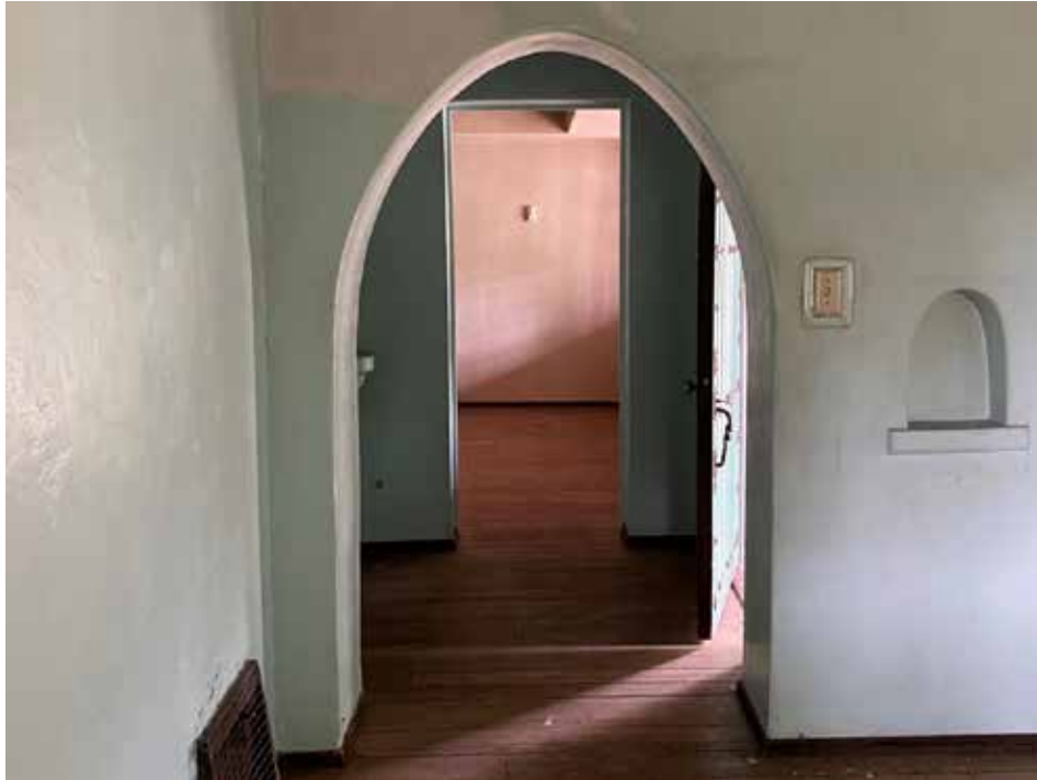
Figure 13. Detail of interior archway, view toward east from living room toward entry hall and dining room.
