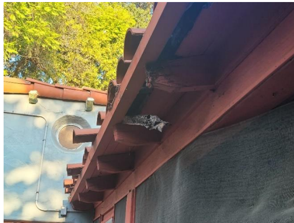
Primary Façade Porch Roof Wood Rot
