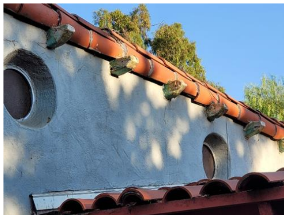
Primary Façade Damaged/Repaired Beams
