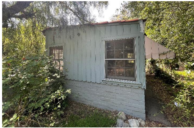
Figure 9J. Western Façade (rumpus room addition; view south) SOURCE: Sapphos Environmental, Inc., 2022
