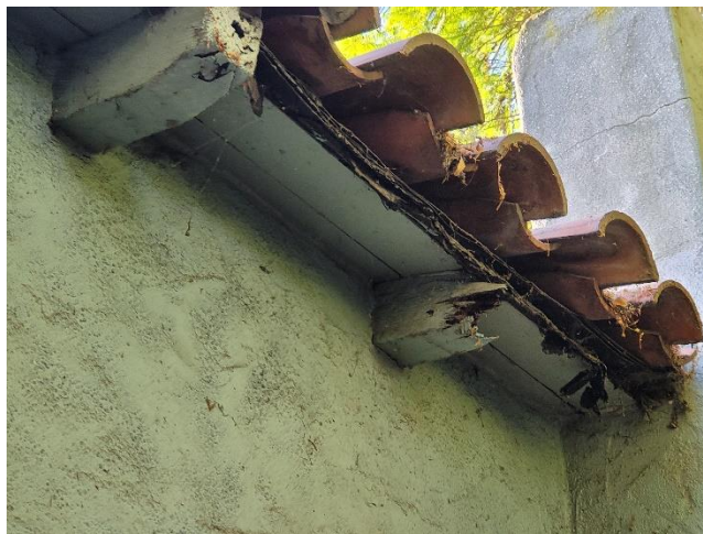
Figure 9A. Western Façade (wood rot) SOURCE: Sapphos Environmental, Inc., 2022
