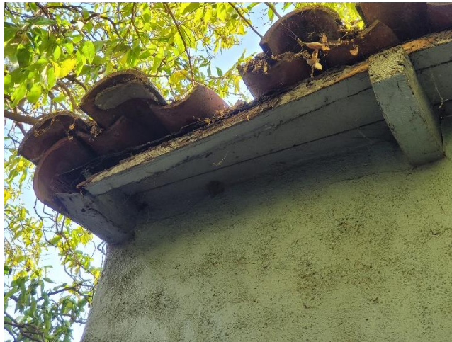
Figure 9C. Western Façade (rafter, wood rot and barrel tile damage) SOURCE: San Gabriel Cemetery Association, 2022
