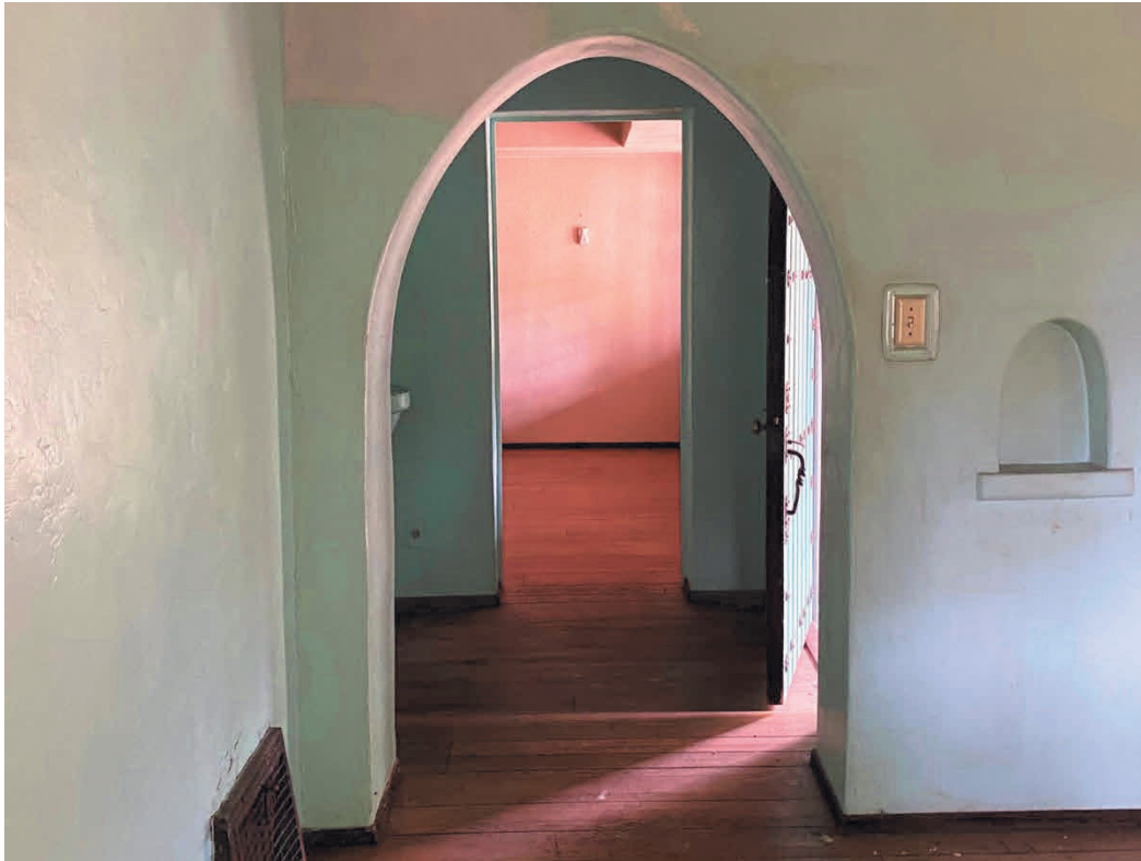
Figure 16. Detail of interior archway, view toward east from living room toward entry hall and dining room.
