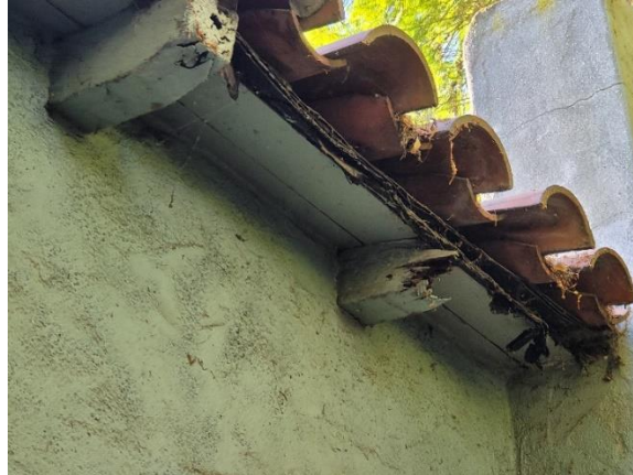
Western Façade (wood rot)
