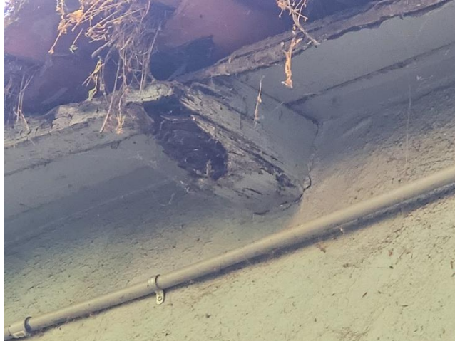
Figure 9B. Western Façade (rafter, wood rot) SOURCE: San Gabriel Cemetery Association, 2022
