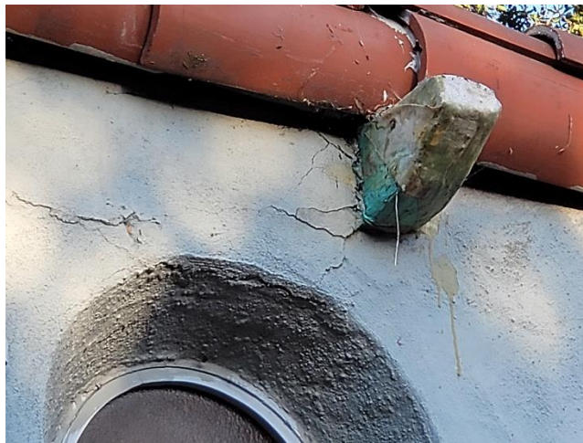
Figure 6K. Primary Façade (damaged beams; view west) SOURCE: Sapphos Environmental, Inc., 2022
