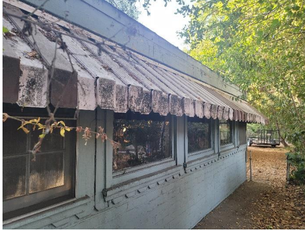
Figure 9I. Western Façade (rumpus room addition; view south) SOURCE: San Gabriel Cemetery Association, 2022
