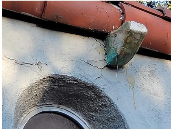
Primary Façade Damaged Beam
