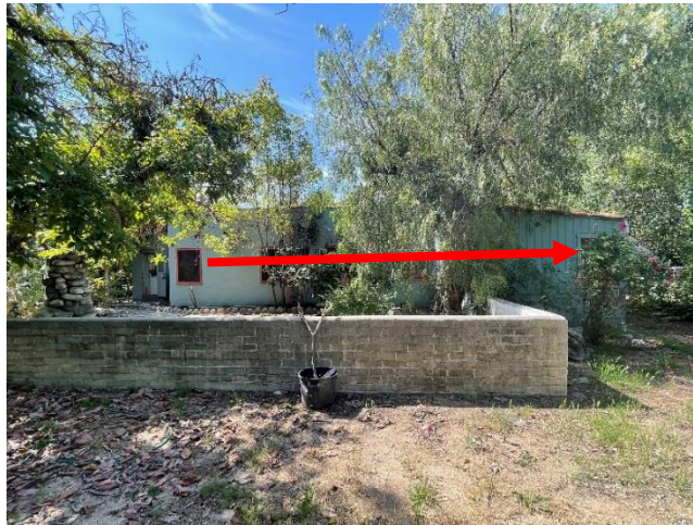
Figure 7B. Northern Façade (view south; arrow identifies 1951 rumpus room addition) SOURCE: Sapphos Environmental, Inc., 2022
