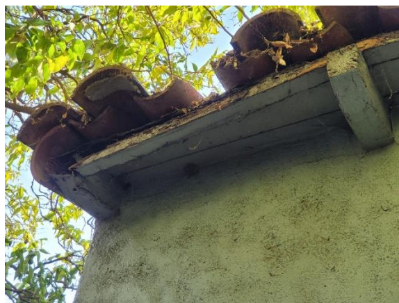
Western Façade (rafter, wood rot and barrel tile damage)
