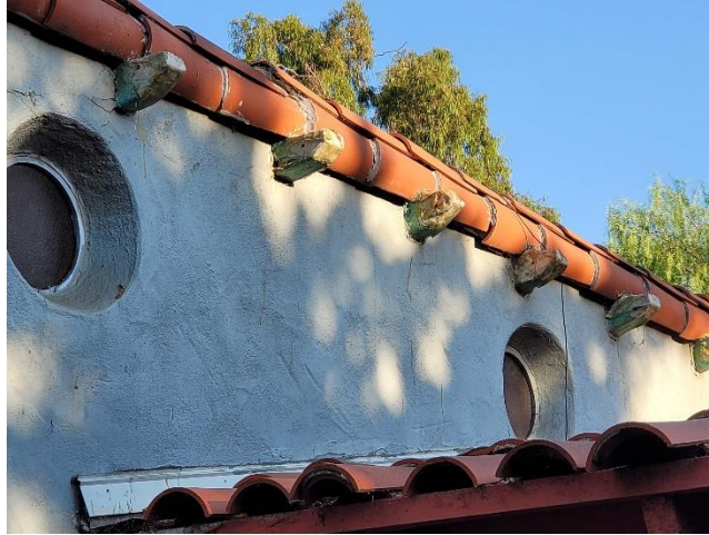
Figure 6J. Primary Façade (damaged/repared beams; view west) SOURCE: Sapphos Environmental, Inc., 2022
