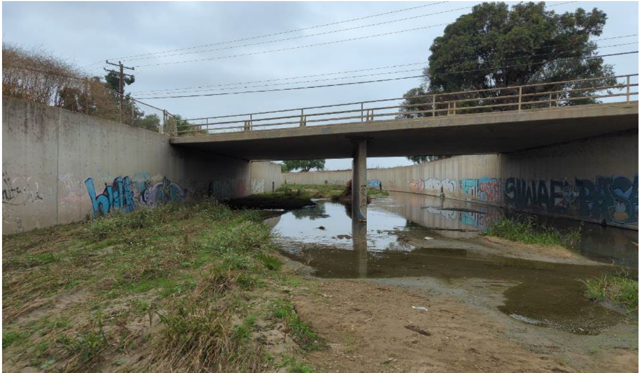
Photograph 23. View of Revolon Slough and the Laguna Road bridge (Aspect: northeast; September 13, 2023).
