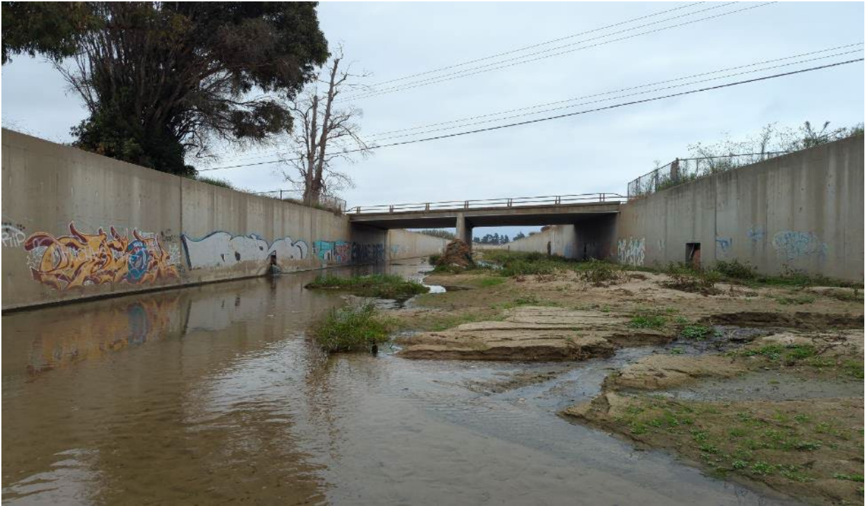
Photograph 21. View of Revolon Slough and the Laguna Road bridge. Note presence of culvert outlets scattered along the concrete side walls of the drainage (Aspect: southeast; September 13, 2023).
