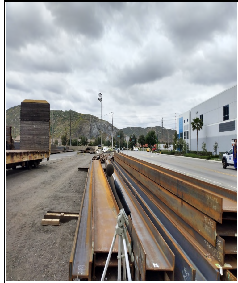
NM (Base Measurement) looking SSW towards Live Oak Ave & Jurupa Ave intersection ( ~470' ).
