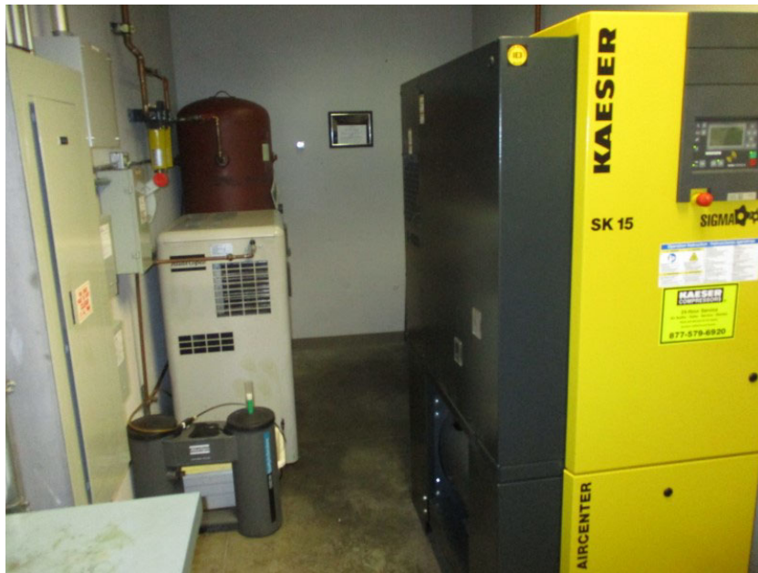
Photo 1. The building air compressor room located in the western portion of the site building. Photograph taken August 22, 2019.
