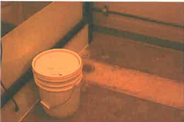
Photo #11: Drain to municipal sanitary sewer system where treated wastewater is disposed of
