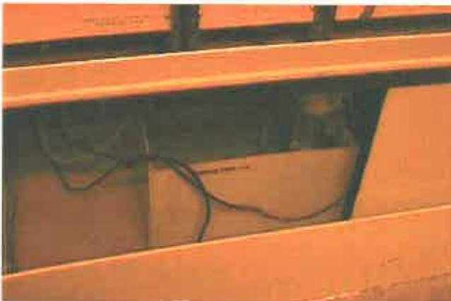
Photo #9: Storage tank for wastewater from used portion of Kepro system — wastewater gets pumped to a series of treatment tanks in PCB Etch Room
