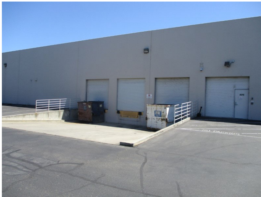
Photo 1. View, facing northeast, of the truck loading area located on the western side of the site building. The truck loading ramp is also used to store solid waste dumpsters. Photograph taken August 22, 2019.
