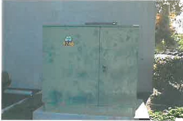
Photo #25: Pad-mounted electrical transformer at Project
