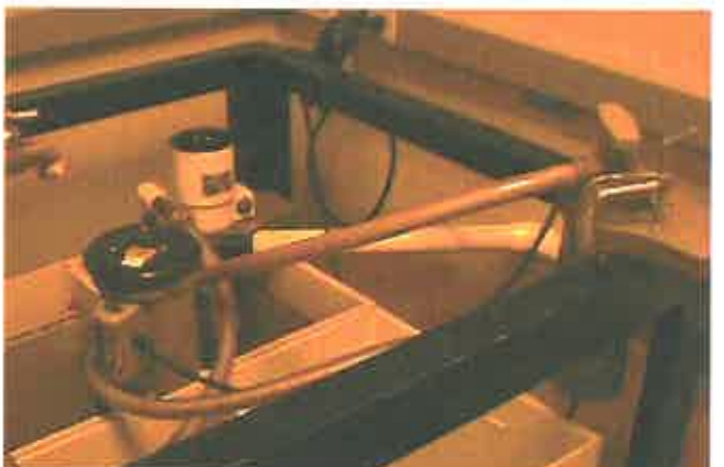
Photo #12: Pump and filter system on wastewater treatment unit
