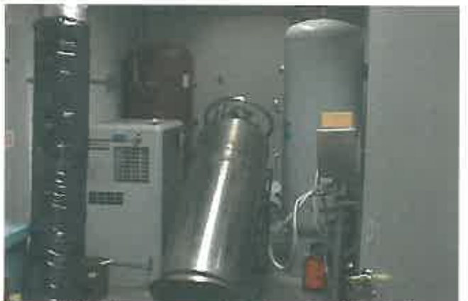
Photo #22: Storage room for carbon dioxide and nitrogen cylinders and tanks
