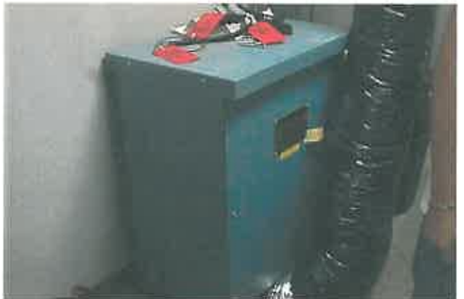
Photo #18: Dry-type transformer at Project
