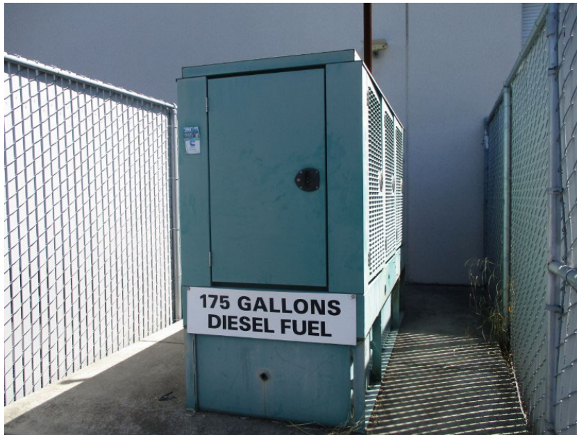
Photo 2. Emergency generator within a fenced enclosure located on the western side of the subject property adjacent to the site building within a fenced enclosure. No staining was observed on the ground surface in the vicinity of the generator. Photograph taken August 22, 2019.
