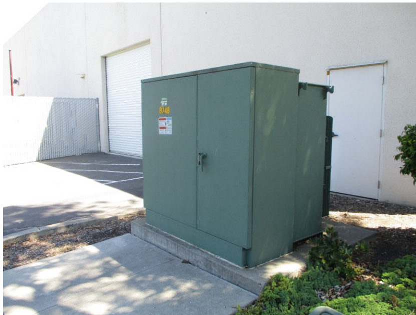
Photo 1. Transformer adjacent to the southwest corner of the subject property building. Photograph taken August 22, 2019.
