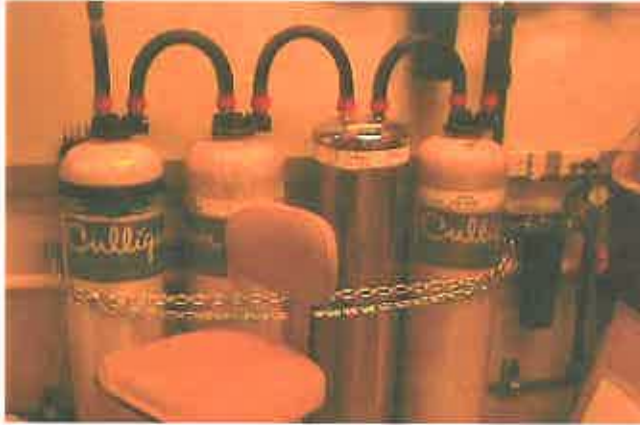
Photo #13: Water deionization system in PCB Etch Room
