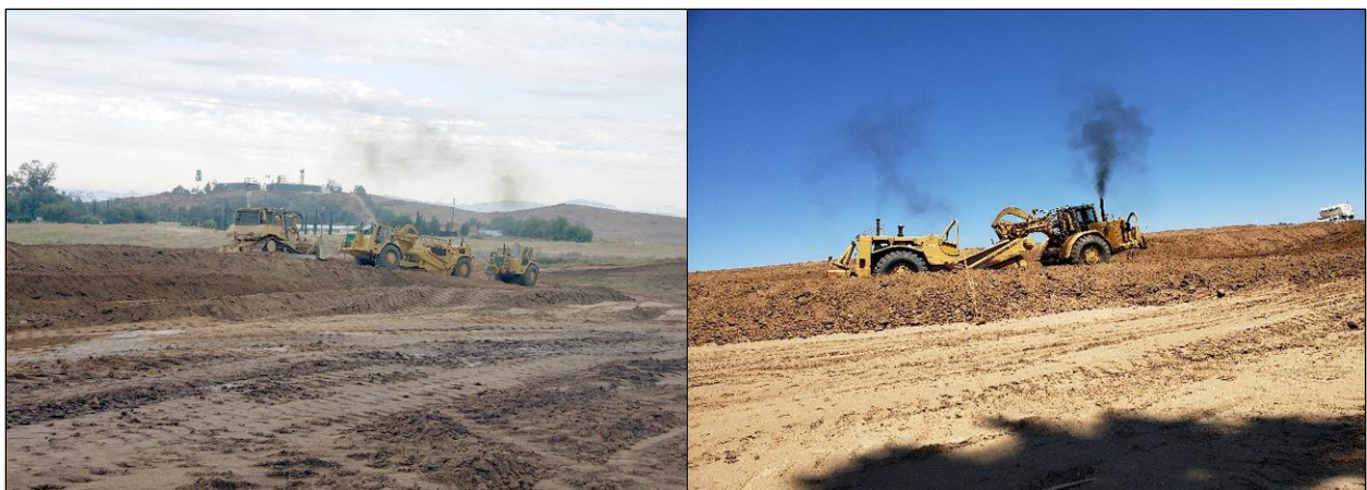
Figure 4. Earth-moving operations in the project area. Left : crews working on a stockpile (view to the southwest, photograph taken on August 6, 2019); right : grading along the slope of the hill (view to the northwest, photograph taken on August 12, 2019).
