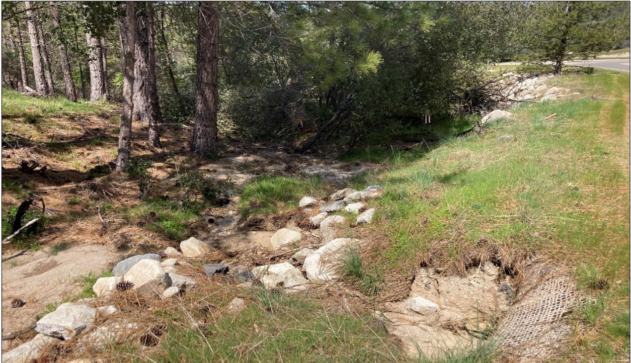
Figure A-7. Photo of an ephemeral drainage crossing the western section of the BSA, facing northwest (downstream).
