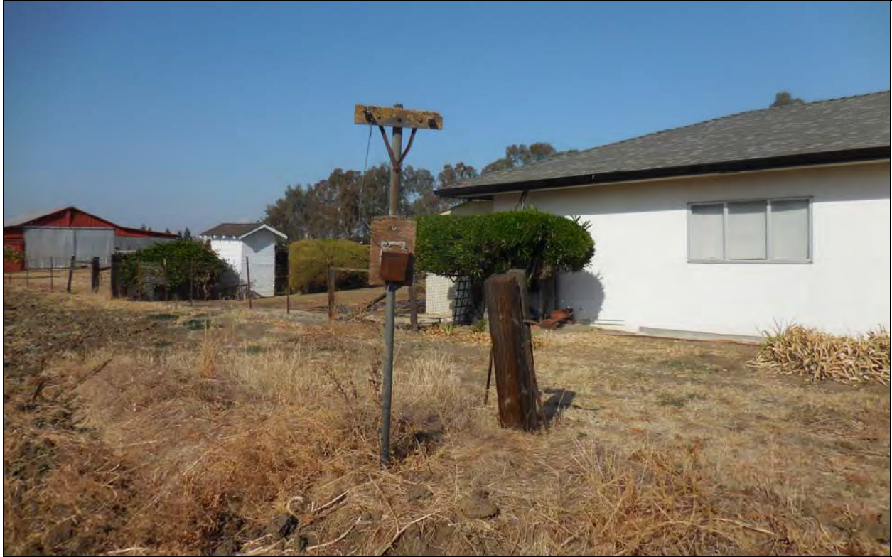
Figure 6: Homart Electric Box, northeast corner of parcel
