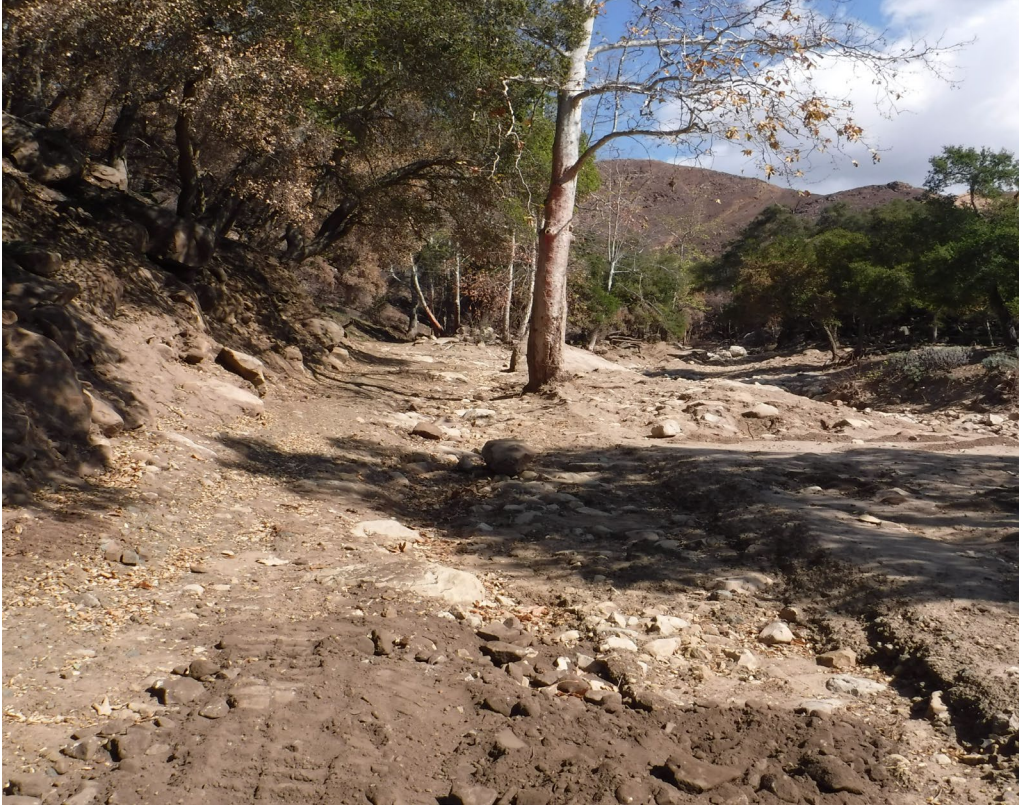
Access road looking northeast from Station 11+00 at start of access road improvements following debris flow on 9 January 2018 that occupied the entire floodplain along this reach. Note proximity of channel (at right) to roadway. 22 February 2018.
