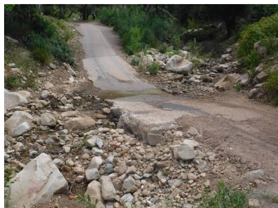
Photograph 4. The existing unpaved dirt access road traverses an approximately 11-foot-wide by 54-foot-long concrete Arizona crossing over Hot Springs Creek. Under the proposed Project, this crossing would be replaced by an 80-foot-long free span bridge.
