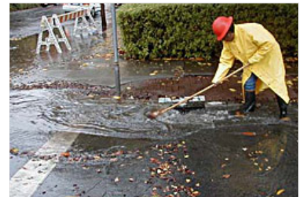
Clogged Storm Drain
