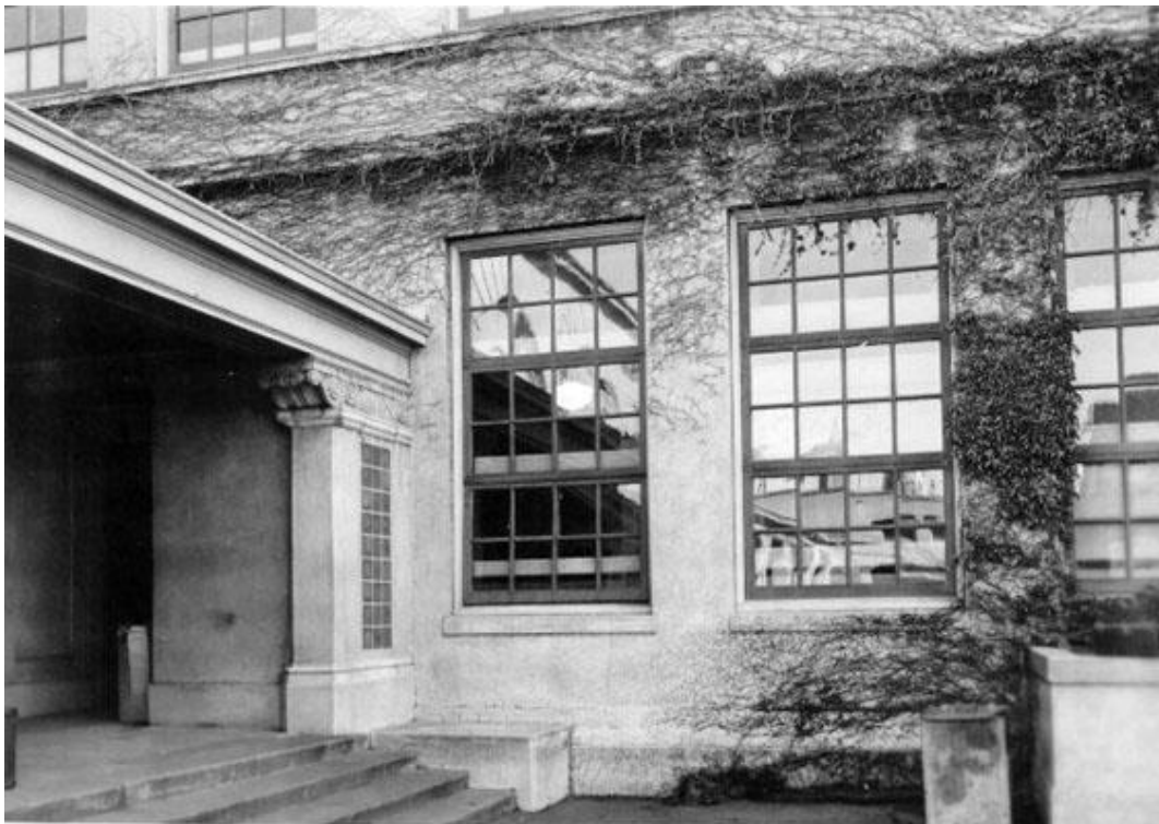
Arcade at west elevation of classroom wing, looking west. Note that original wood — windows are still present. San Francisco Public Library.
