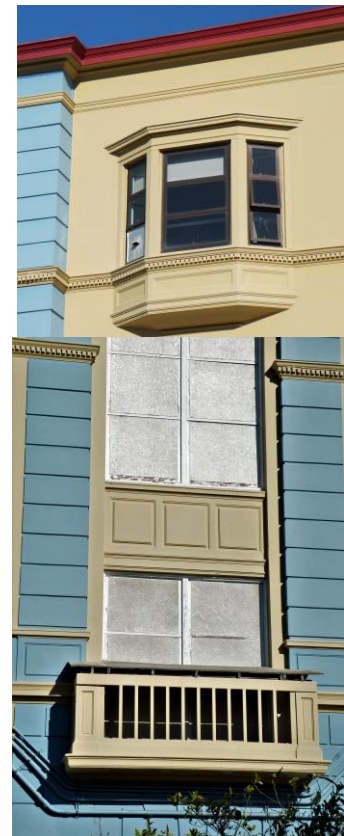
The bay window and the balconette on the south façade of the classroom wing are not classical devices, but they exhibit the articulation used by the Classical Revival style. Knapp Architects photos.
