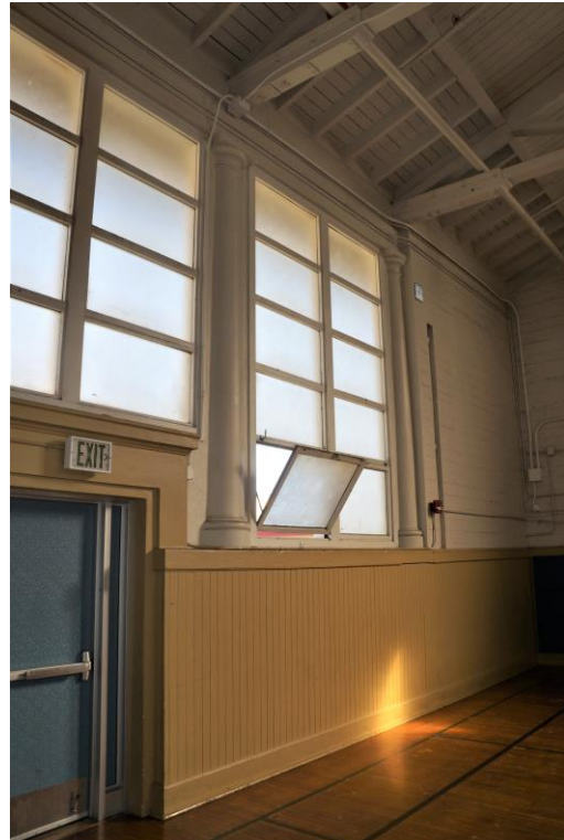
When windows were installed, the columns were left intact and are visible on the interior and exterior. Knapp Architects 2022.
