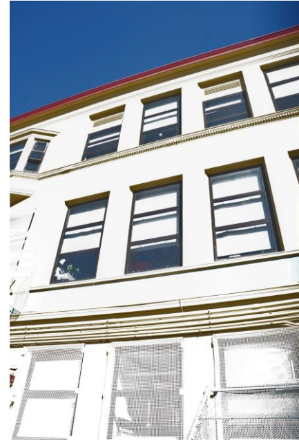
Metal windows replaced the original wood units on the south façade of the classroom wing and heavy security screens were added.
