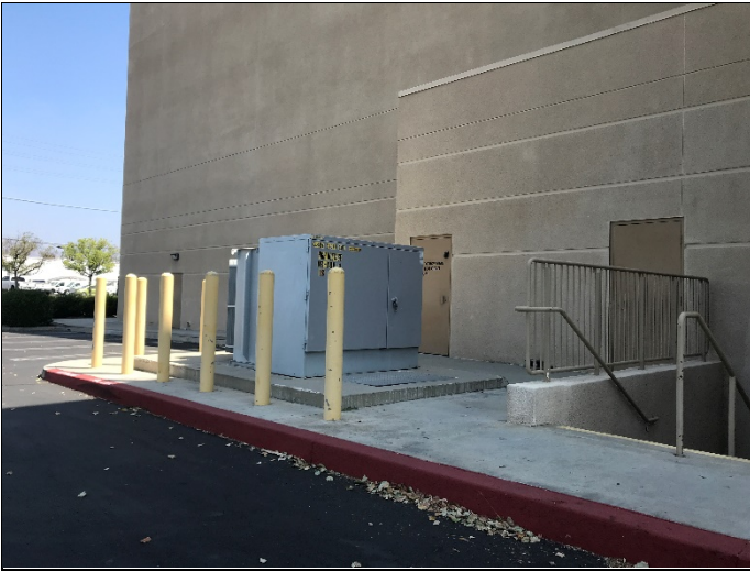
13. Pad-Mounted Transformer along the Western Wall of the Property
