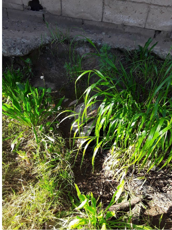
Photo 3. Drainage pipe that undergrounds and leads into daylight portion of Feature 1. March 17, 2022.
