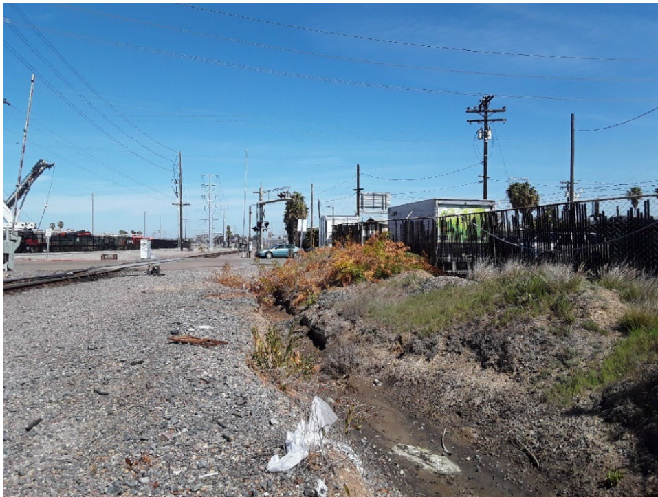
Photo 8. Feature 2 – Manmade brow-ditch south of Civic Center Dr. and Tidelands Ave, underground crossing pictured. March 17, 2022.
