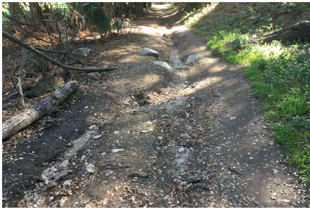
Photo Location 5. January 21, 2022. View of trail, facing south. Erosion was observed on trail that is apparently the result of water that has flowed along trail.
