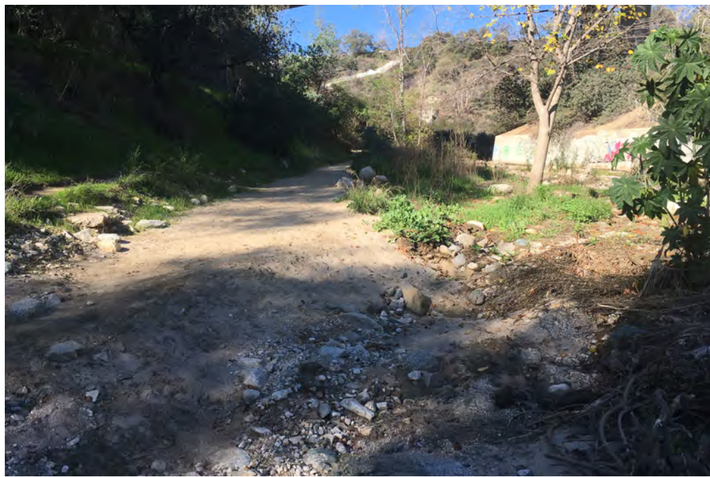
Photo Location 8. January 21, 2022. Ground level view of trail as it runs along the western bank of Arroyo Seco. Trail is 2-3 feet above the grade of the adjacent stream bottom.
