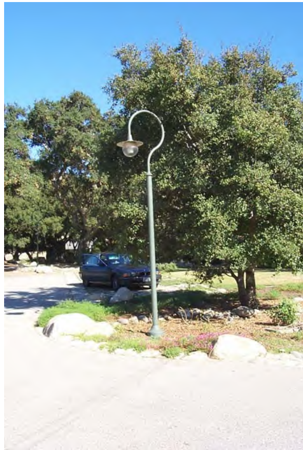
Figure 11-2 The La Casita parking lot light shown here is an example of a desired fixture for other areas in the Arroyo Seco.
