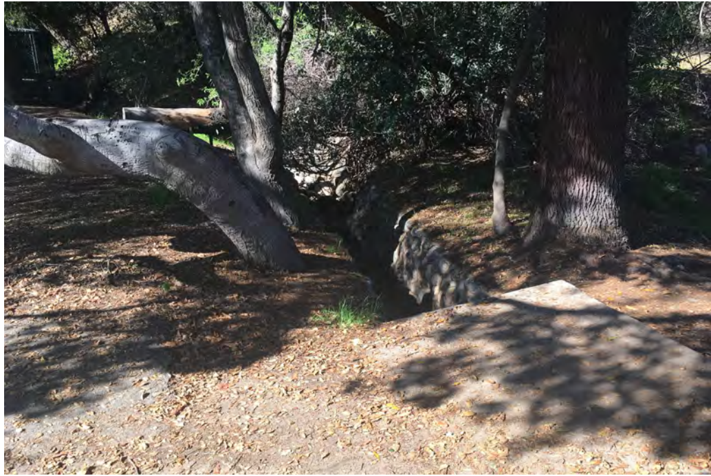
Photo Location 1. January 21, 2022. View of Feature A, a hardened drain with vertical sides. The concrete slab in foreground serves as a bridge across the drain.
