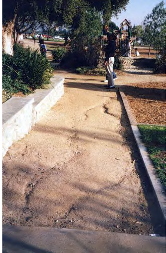
Figure 8-3 An example of erosion on a sloped decomposed-granite pedestrian path.
