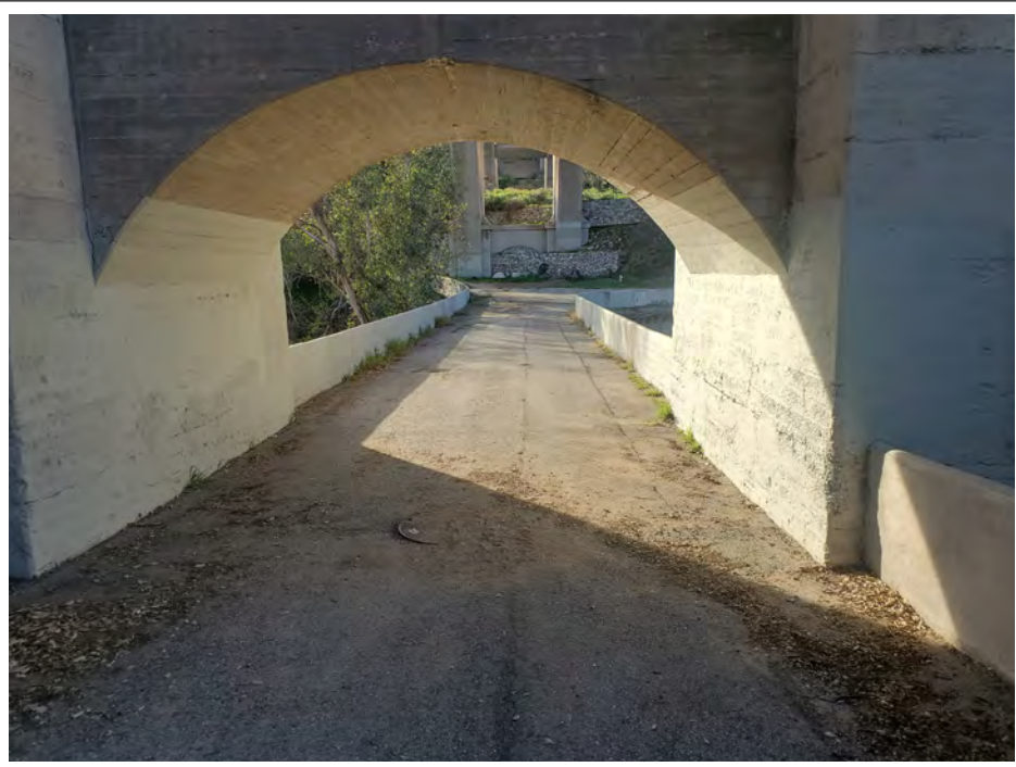
View of the existing pedestrian bridge under the Colorado Street Bridge along the Lower Loop Trail.
