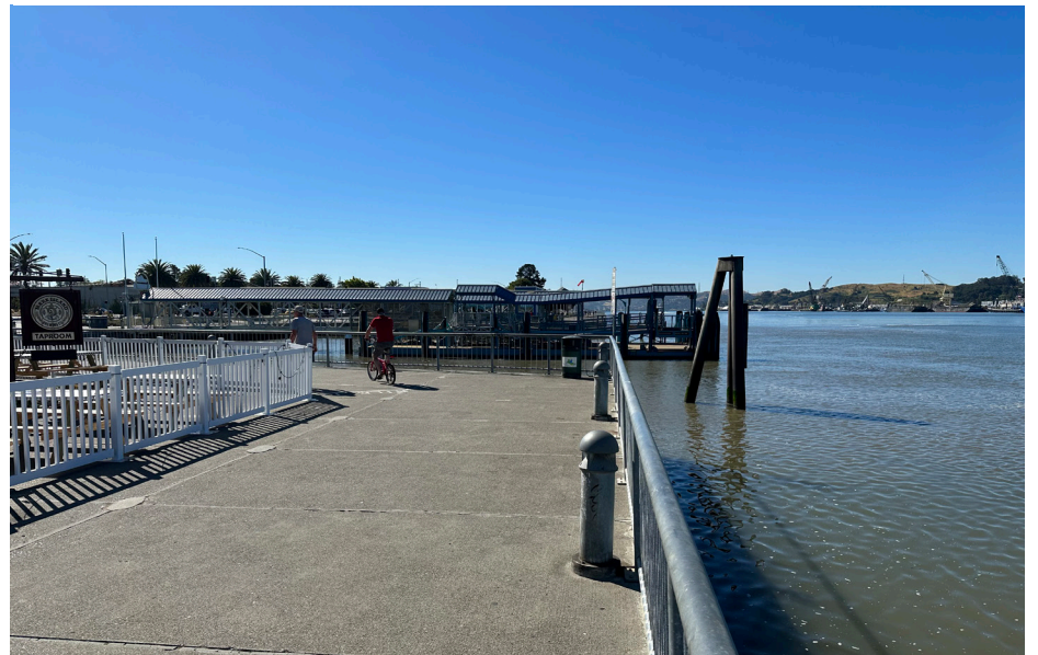
View facing south; See other steel solphin to be removed on northern side of float.
