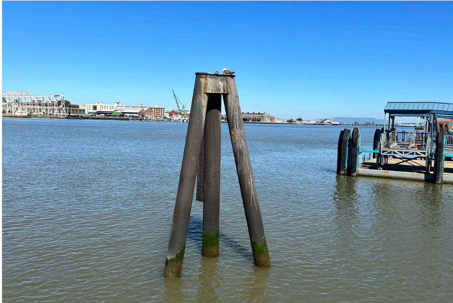
Steel dolphins in basin area on either side of terminal to be removed.
