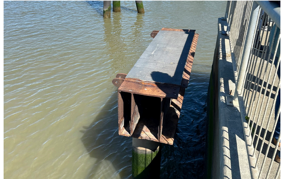
Existing temporary terminal support dolphin and piles to be removed pending Alternative chosen.
