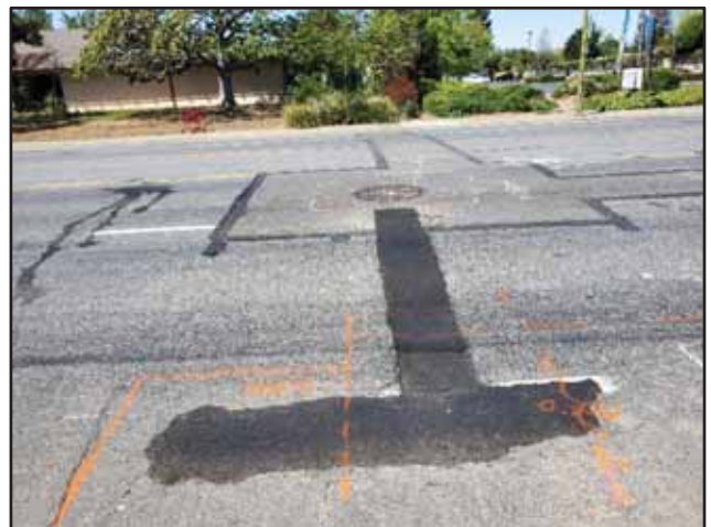
Photograph 10: A T-shaped asphalt patch was observed on Union Avenue adjacent to the southwestern corner of the subject site indicating the presence of sewer lines.
