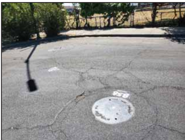
Photograph 11: Two storm/ sewer drain manhole steel covers labelled "857" (background) and "858" (front) were observed at the intersection of Byron Way and Jennifer Way adjacent to the north of the subject site.
