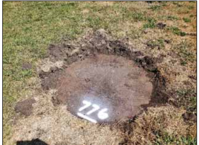
Photograph 4: A manhole steel cover labelled "776" observed on southeast corner of the site. The purpose of the manhole is unknown.
