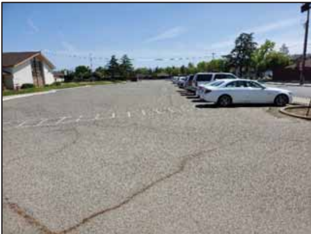
Photograph 7: Straight cracks were observed in the parking lot of the adjacent Metzler School property, possibly indicating the presence of an underground sewer line.
