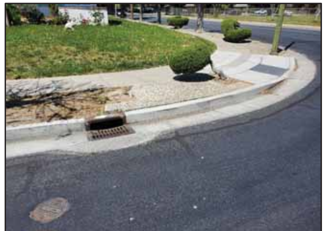
Photograph 8: Stormwater drain found at the intersection of Jennifer Way and Cambrainna Drive.
