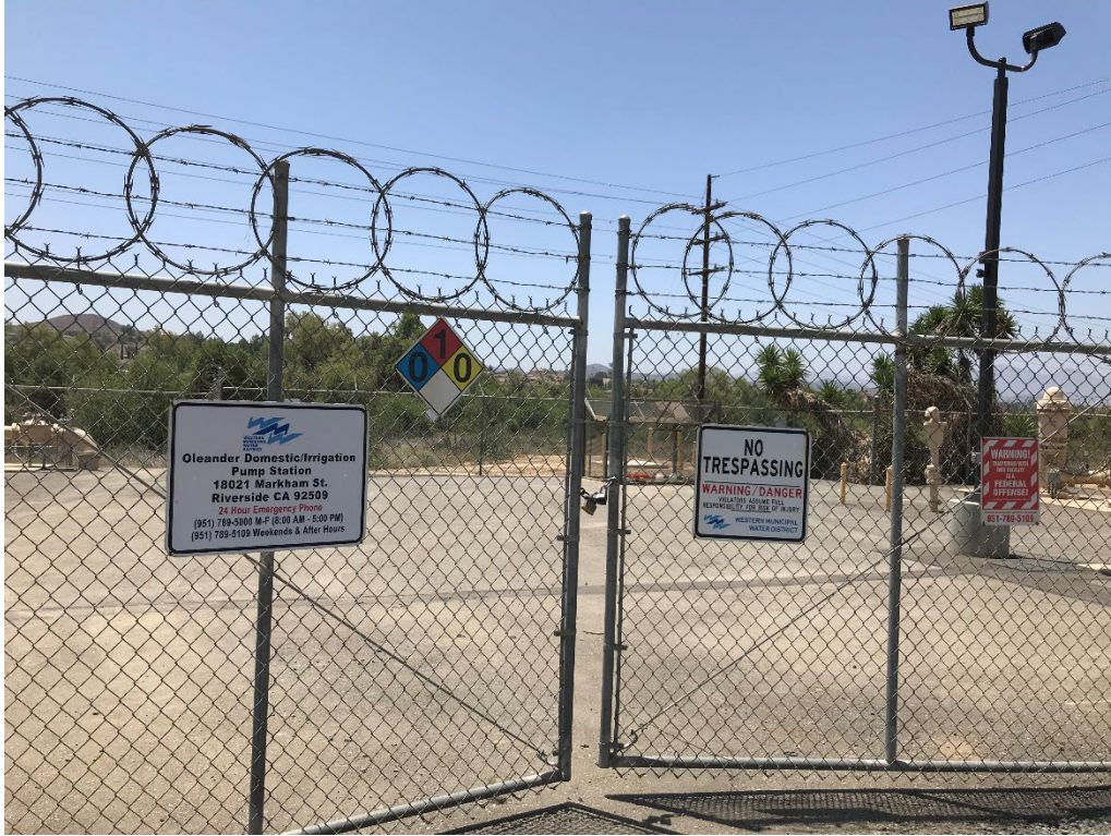
Site 1 – Oleander Domestic/Irrigation Pump Station (18021 Markham St, Riverside, CA). Photo facing south.
