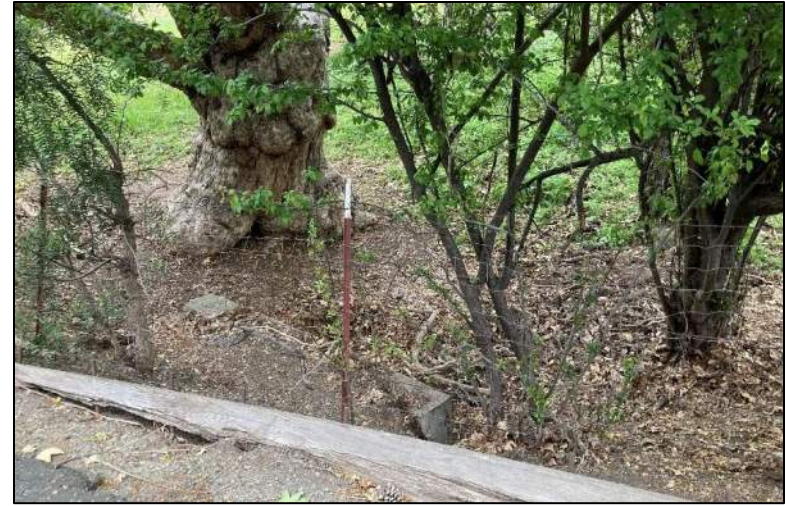
Photograph 2. Culvert and drainage channel located immediately outside the facility entrance. Photo taken on March 25, 2022.
