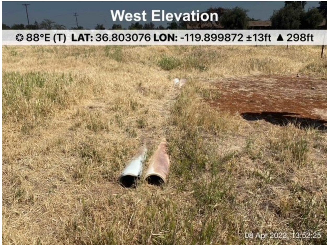
Photo 8: Dilapidated Irrigation Equipment 1
