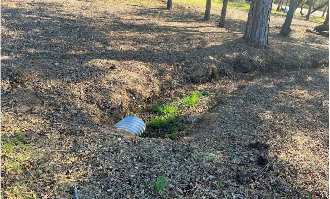
Photo 5. Downslope side of the access road across from the side slope wetland vegetation. Road cut appears to be partly holding back hydrology on upslope side.
