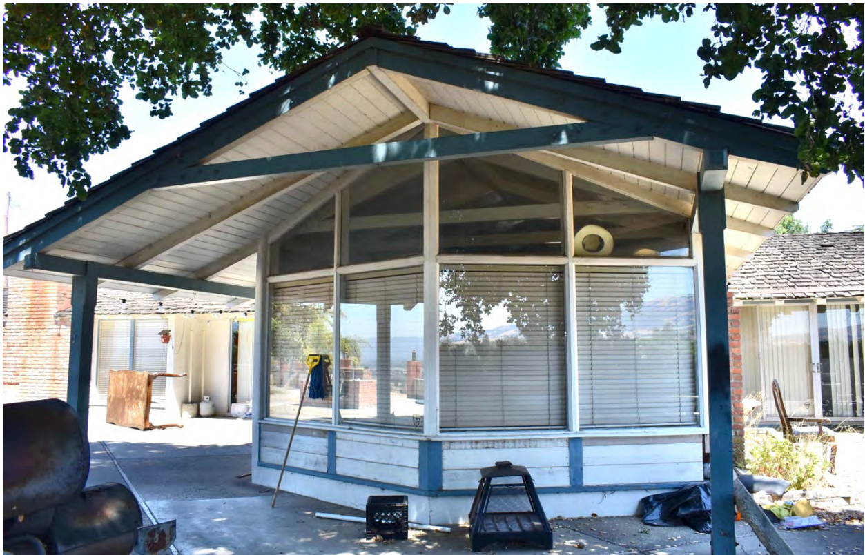
South façade of south wing with angled windows and gable roof extension
