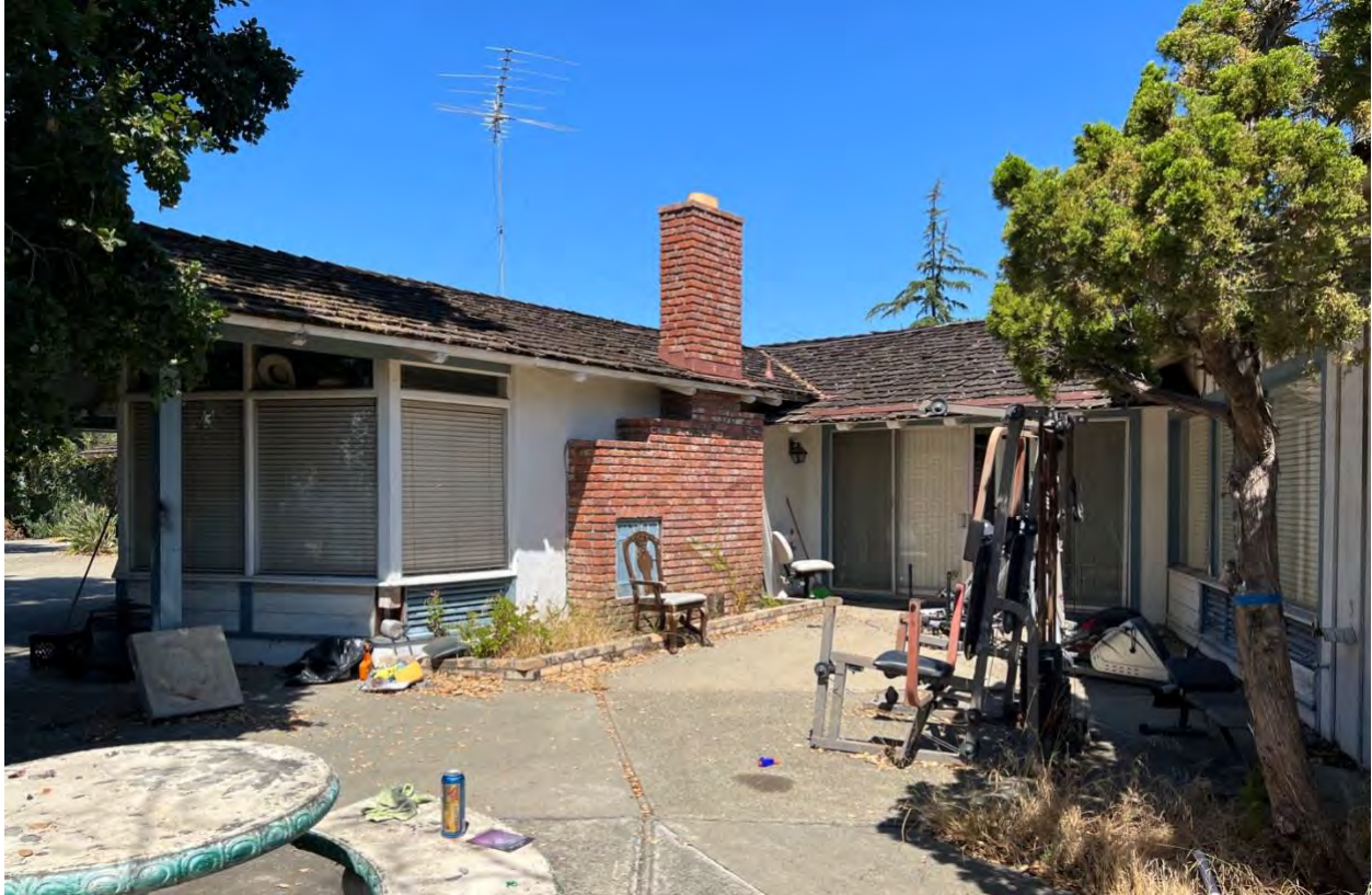
Figure 19: South façade of eastern part of main wing, south wing to the left, east wing to the right
