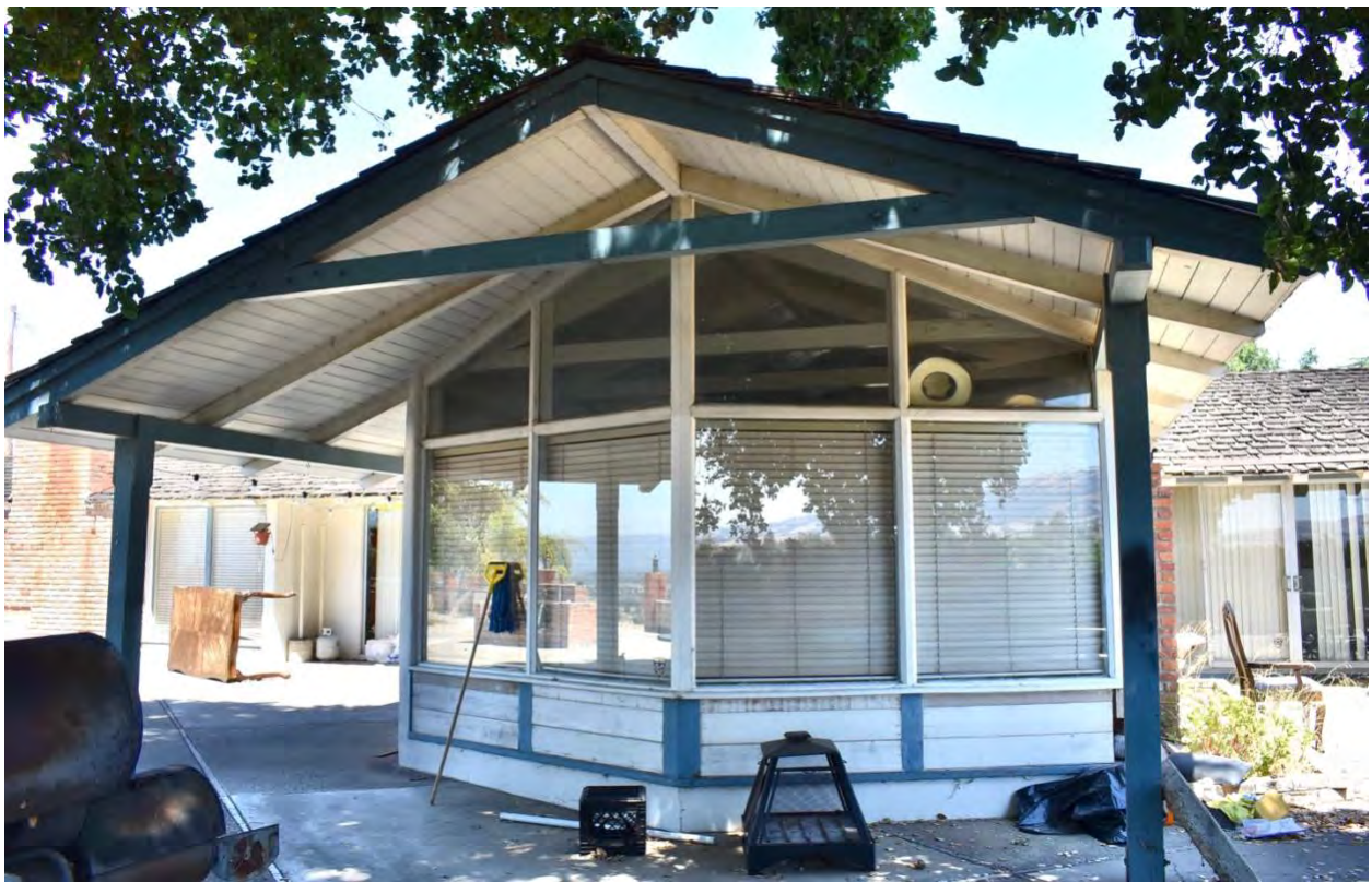
Figure 22: South façade of south wing with angled windows and gable roof extension
