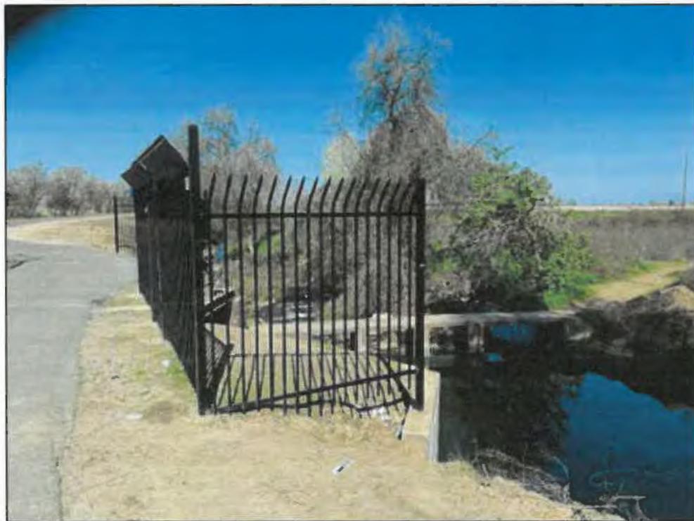
Figure 14. Gate and trail located over Modoc Ditch headgate structure with checkgate (at right). View toward northwest.
