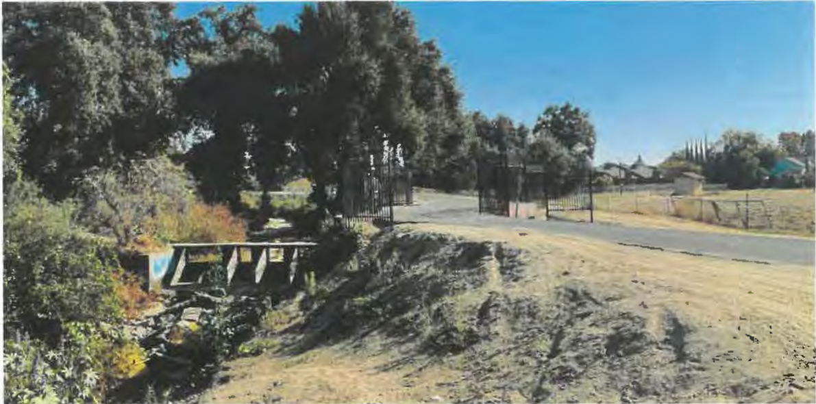
Photo 1: Facing east on Levee Drive looking at the concrete diversion structure in the anabranch of St. John's River. Litter in the form of yellow shopping carts can be seen on the bottom left of the photograph. Modoc Ditch is on the right side of the photograph. Field in background.
