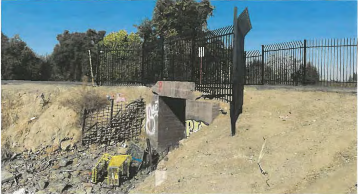
Photo 8: Debris in Modoc Ditch. Looking north.
