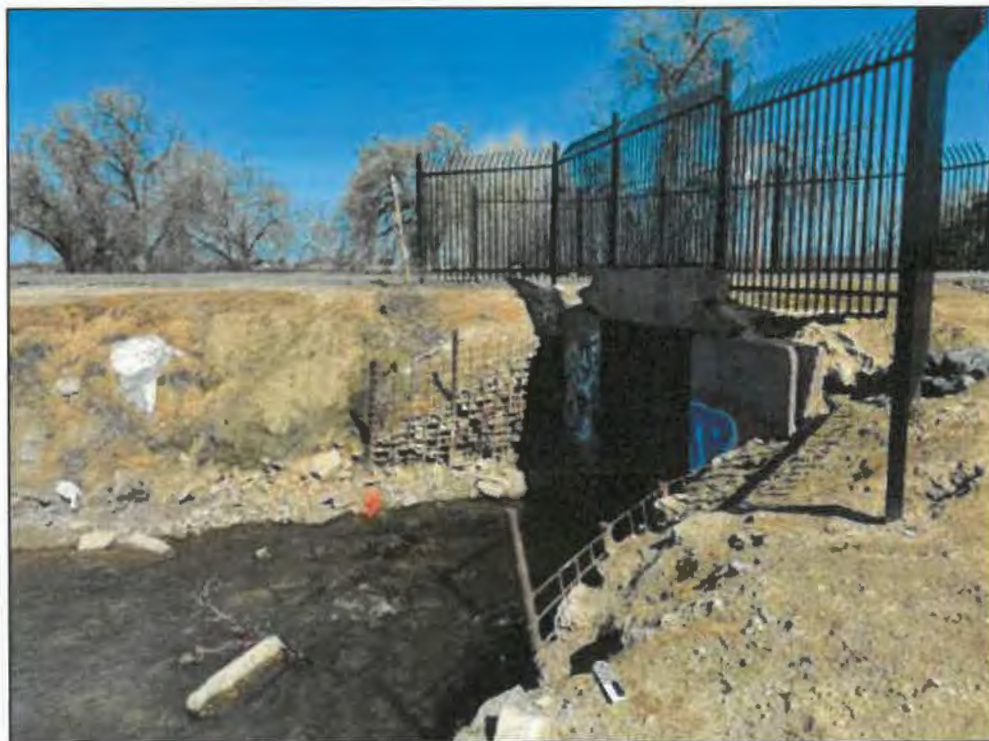
Figure 12. Modoc Ditch headgate structure with metal rebar fencing to protect against side wall erosion, view toward north.
