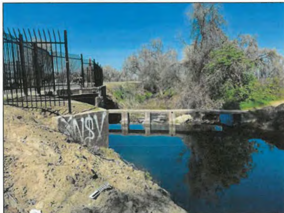
Figure 10. Modoc Ditch checkgate (at center) with headgate to culvert (at left) below bars. View toward northwest.
