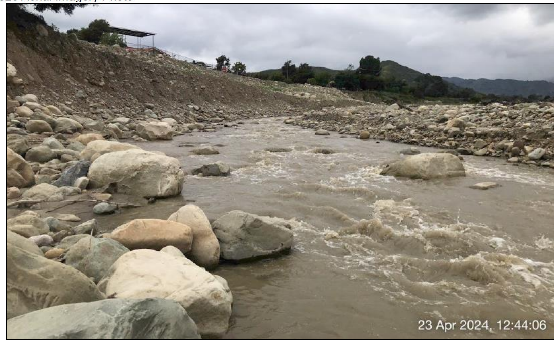
Taken 4/23/2024 - along Santa Paula Creek showing a steep slope (along the west bank) where the residential properties are located and no existing vegetation along with section of the creek.
