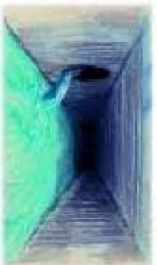
Underground storm drain
