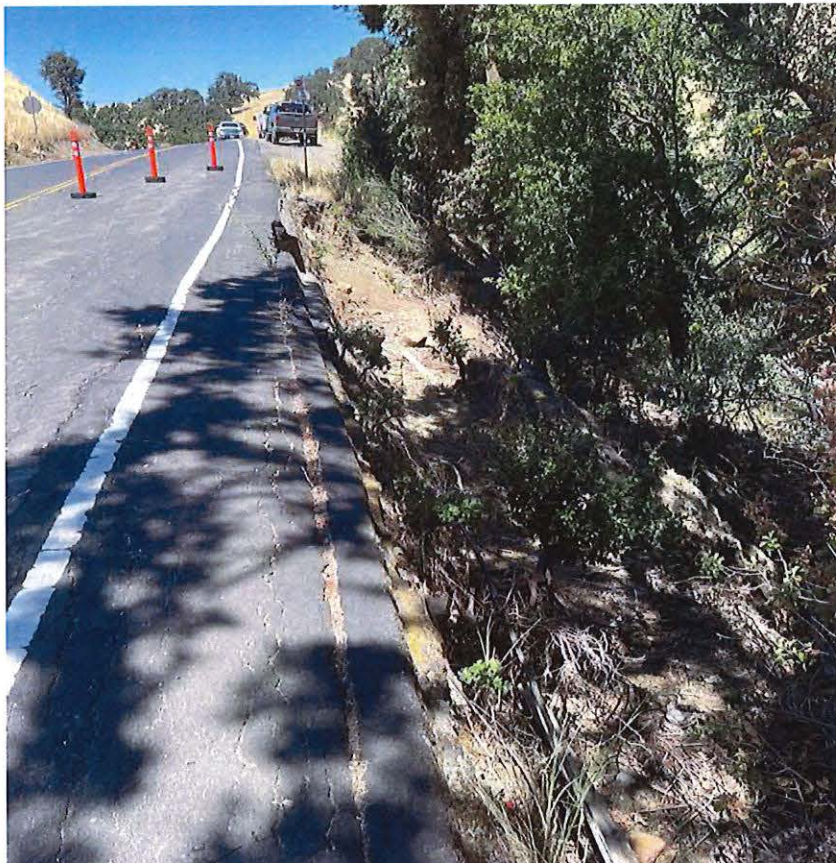
Photo 2. Damage along Northbound Los Vaqueros Road (facing north)
