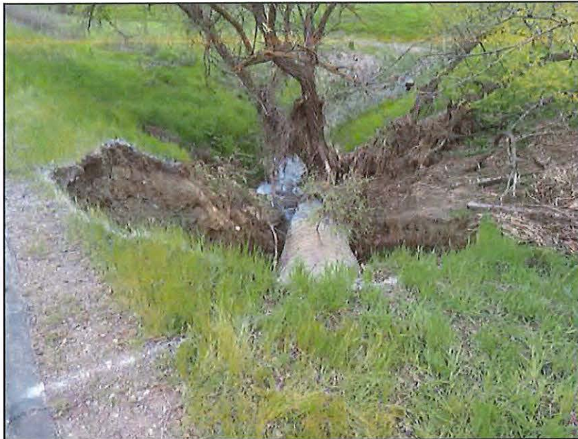
Photo 1. Damage to Culvert 24 (upstream side, taken from southbound Los Vaqueros Road)
