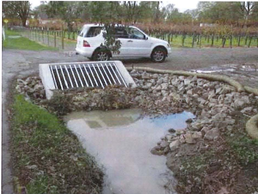
Photo 5. Example of Angled Debris Rack at Culvert Inlet
