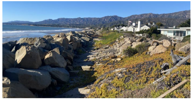
The Sandyland Shoreline Protection was improved in 1983. These improvements raised and widened the crest, increased the armor rock size, and extended the rock footprint seaward and landward.
