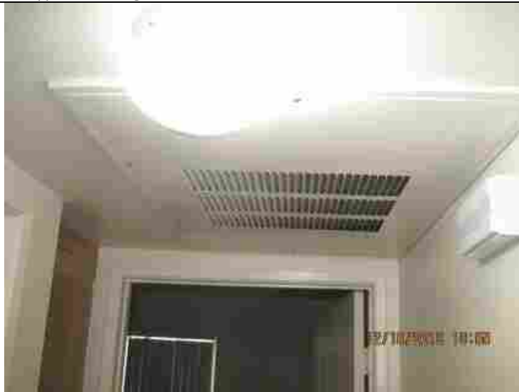
11- Typical Fan Coil Heat Pump
