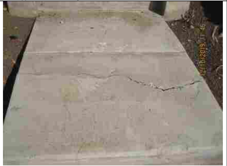
52- Typical Concrete Cracking
