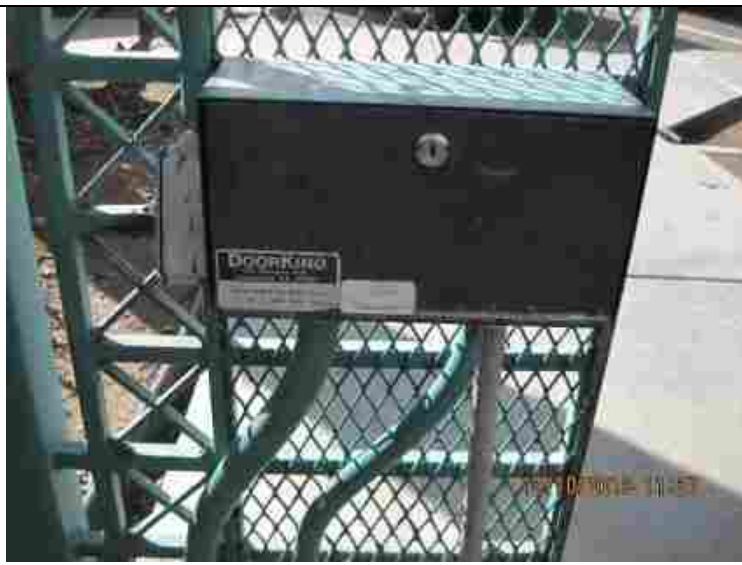
31- Telephone Entry System
