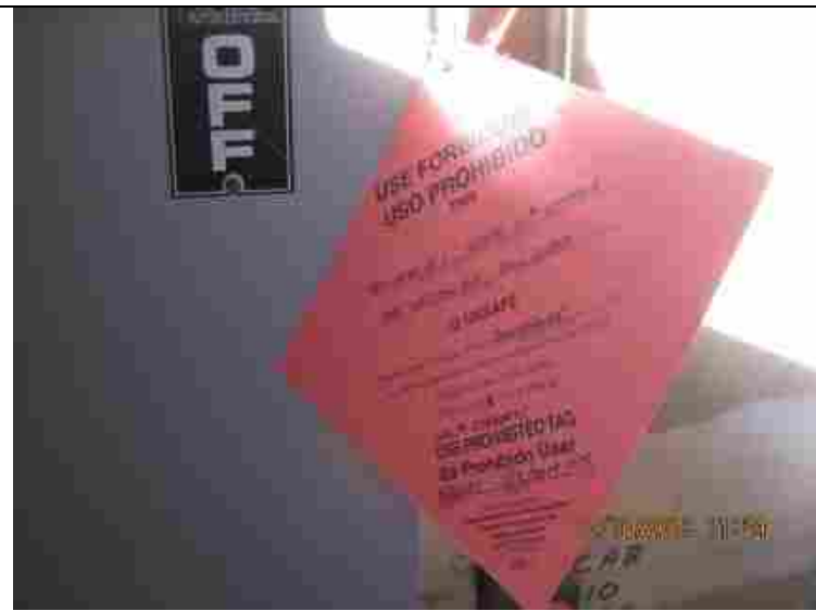
19- Elevator Equipment - Use Prohibited Tag
