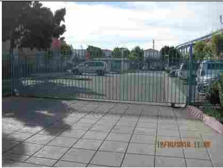
35- Automatic Security Gate
