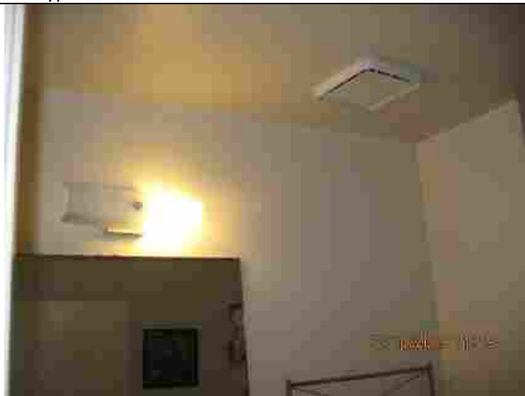
17- Typical Bathroom Exhaust Fan
