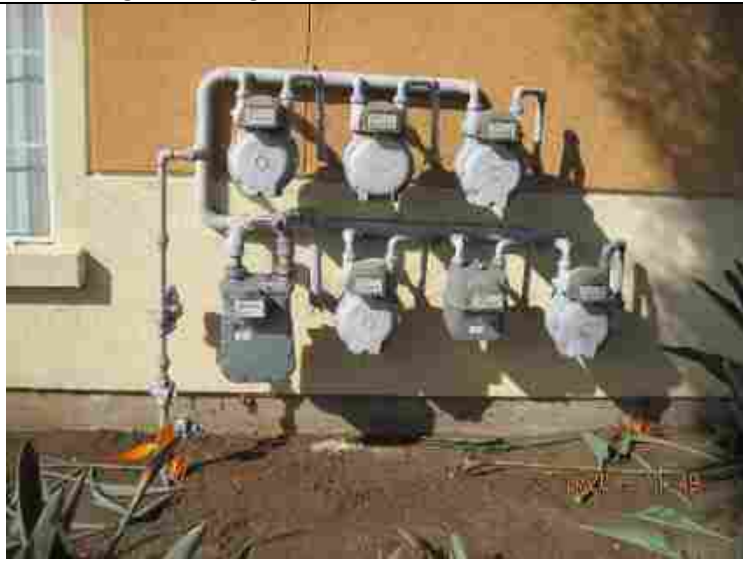
53- Typical Gas Meters
