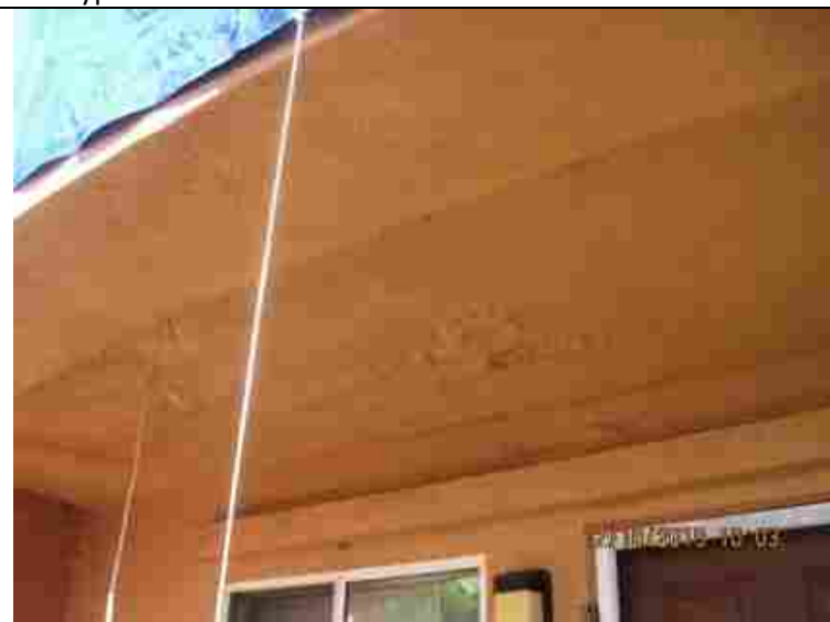
23- Blistering Stucco Ceiling
