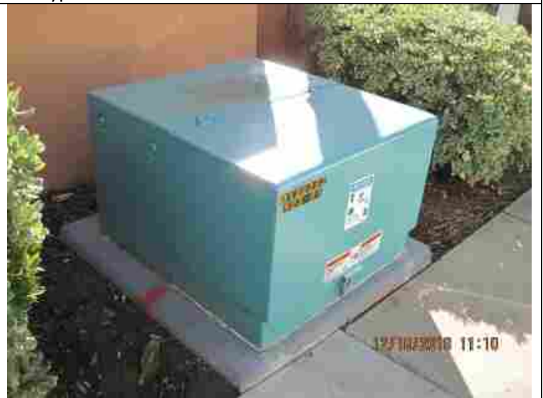
40- Typical Pad-Mounted Transformer
