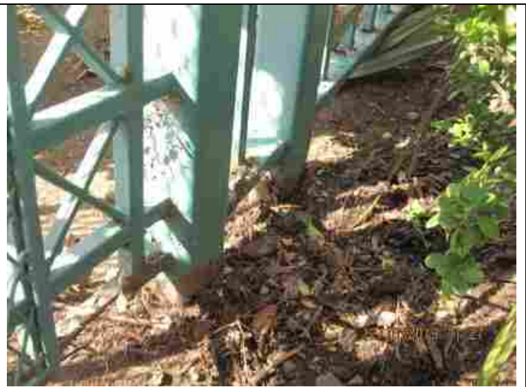
20- Rust and Corrosion _ Wrought Iron Gates
