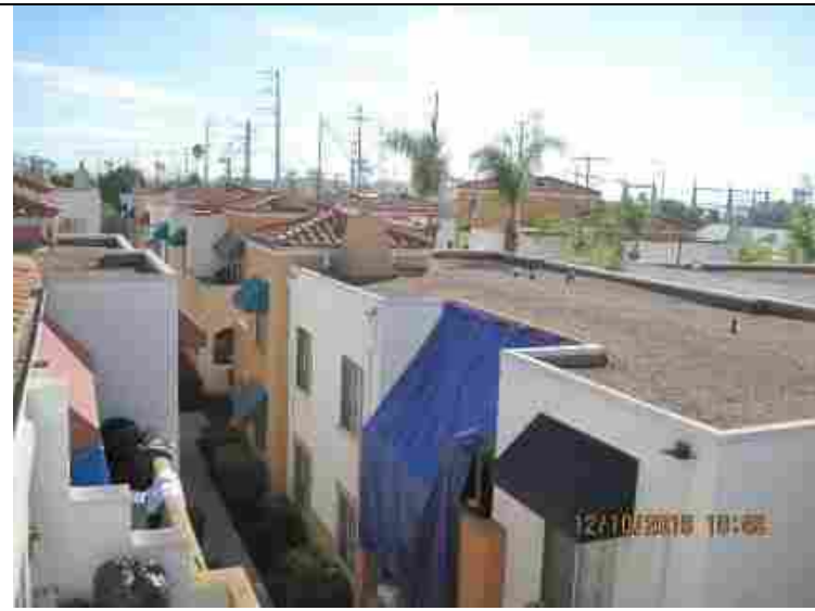
25- Blue Tarp Covering Balcony
