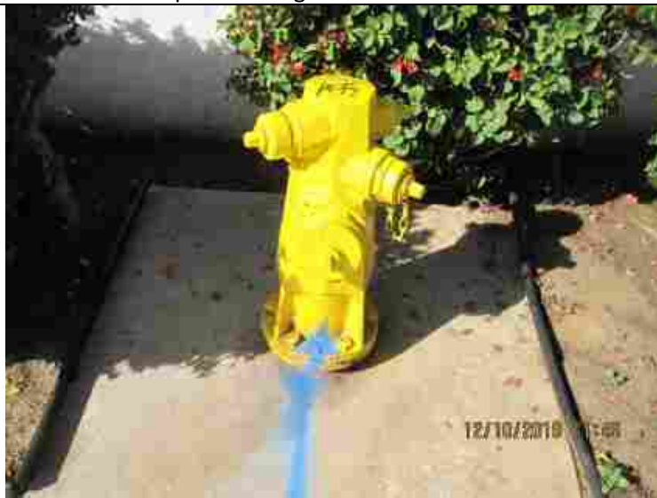
45- Typical On-site Fire Hydrant
