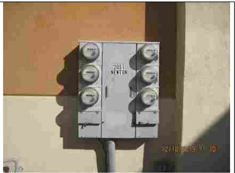
38- Typical Electrical Meters
