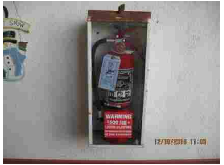
50- Typical Fire Extinguisher
