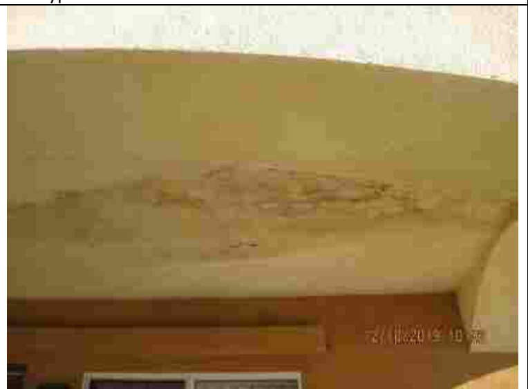
24- Stucco Soffit surface - Water Damage
