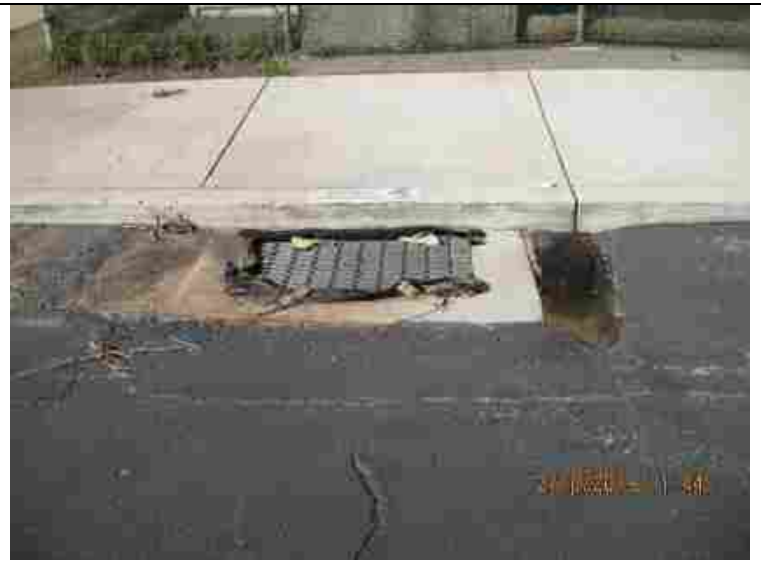
44- Typical Stormwater Drainage Inlet
