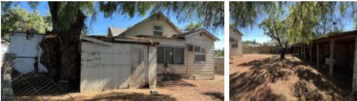
Figures 20 and 21. North elevation of Building 4 on the right and the shed on the left (August 2022).
