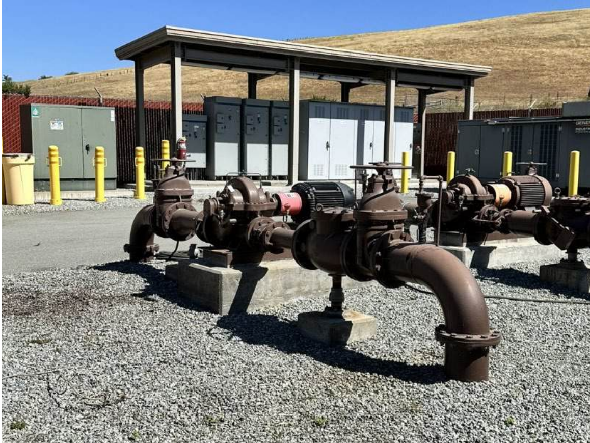
Figure 2-3: 2.25 MGD Raw Water Pump Added to the Existing Raw Water Pump Station (RWPS)
