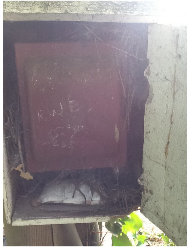
Well Pump Fuse Disconnect
