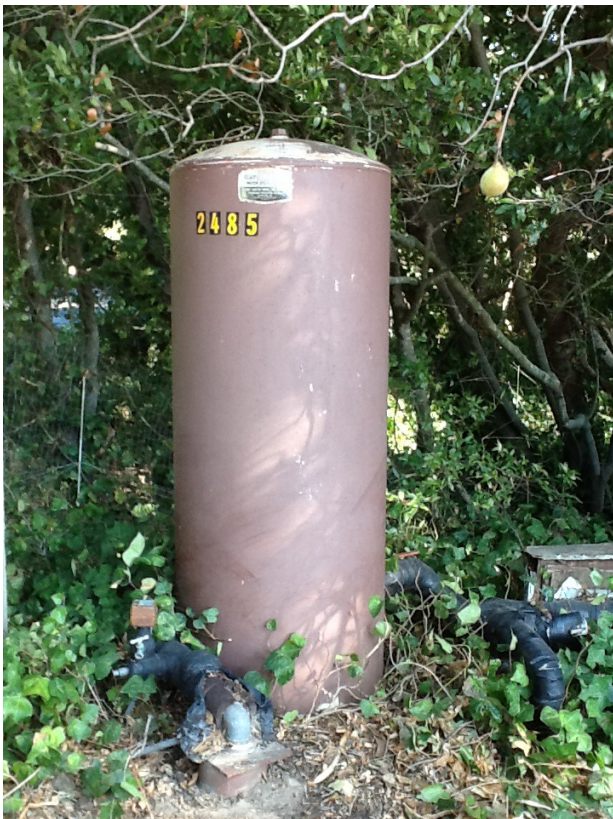
Well Pump Pressure Tank
