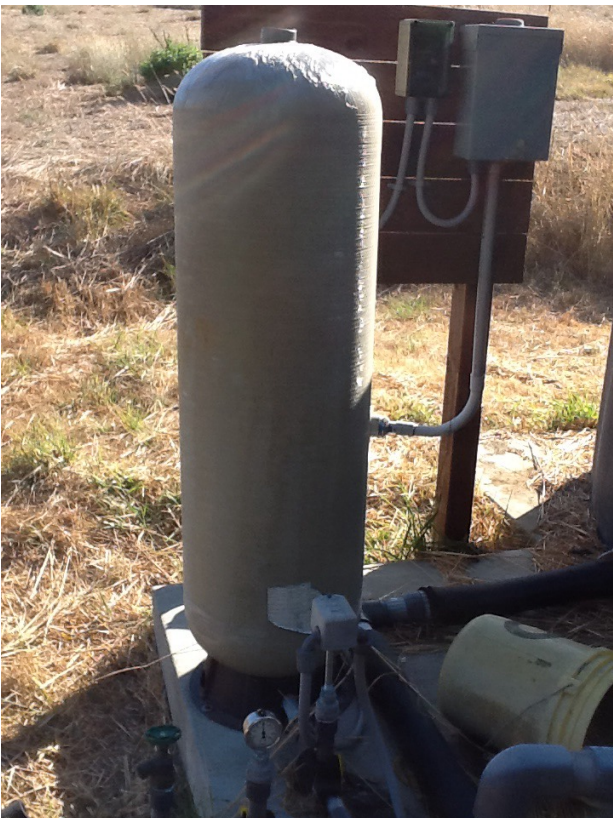
Booster Pump Pressure Tank
