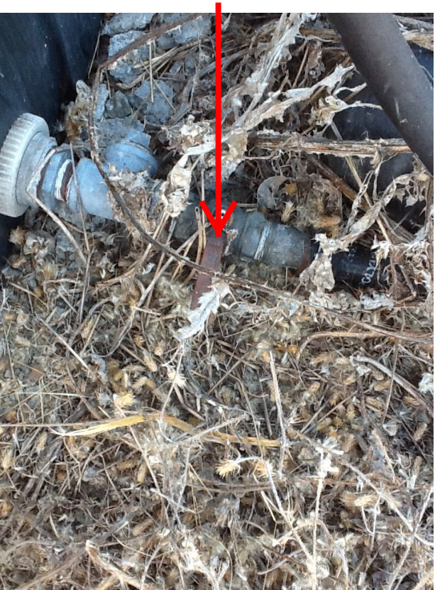
Upper Tank Outlet Valve
