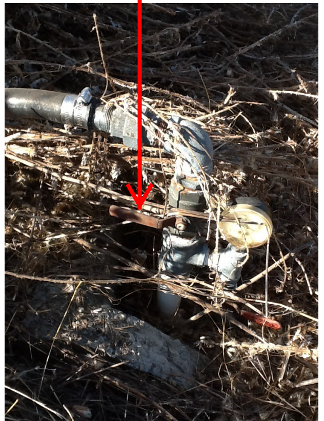
Upper Tank Fill Valve
