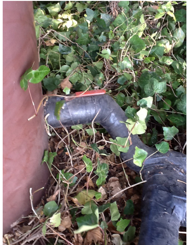
Main Shut Off Valve
