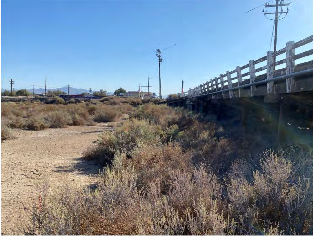
Photo 3. Overview of north face of bridge from within the Mojave River Channel. View facing northeast.
