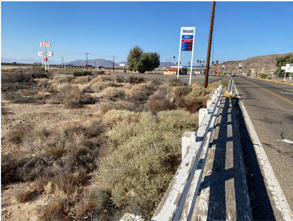
Photo 4. View of Mojave River Channel along the south edge of Bridge No. 54C-0127 with the modern Mobil gas station in the background. View facing southwest.
