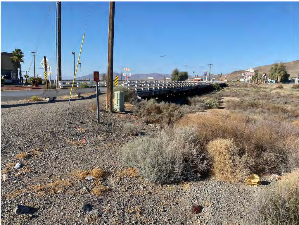
Photo 2. Overview of APE near the northeastern wingwall of the existing bridge. View facing southwest.
