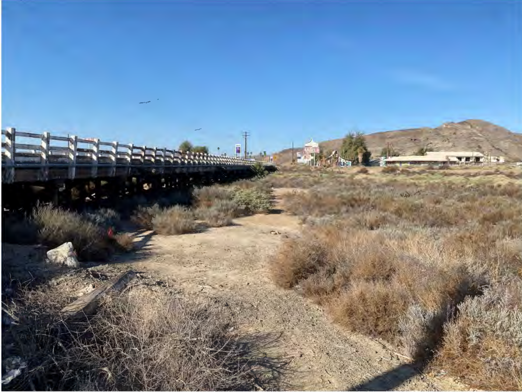
Photo 1. Overview of northern profile of Bridge No. 54C-0127 from within the Mojave River Channel. View facing southwest.
