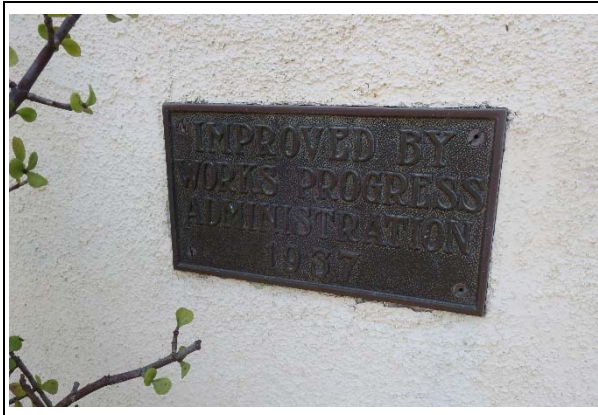
Building B, detail of Works Progress Administration Plaque on primary (north) façade (ARG, 2021)
